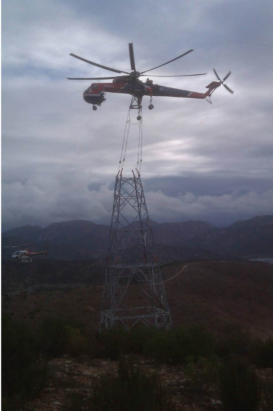
Sky crane installing a section of the tower at CP40-2. Photo courtesy of Joel Herrmann.
