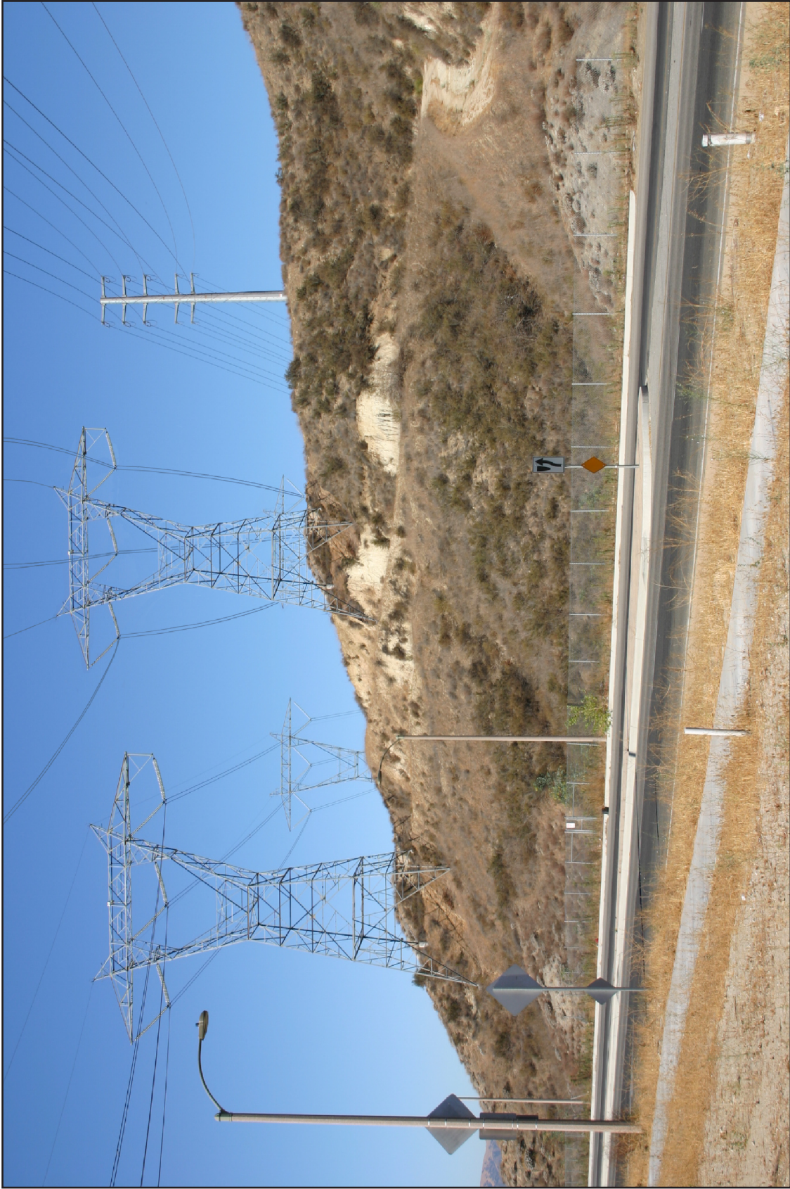
© Alternative 2 - 500 kV single circuit transmission line replacement as seen from KVA Seg 1-9.
