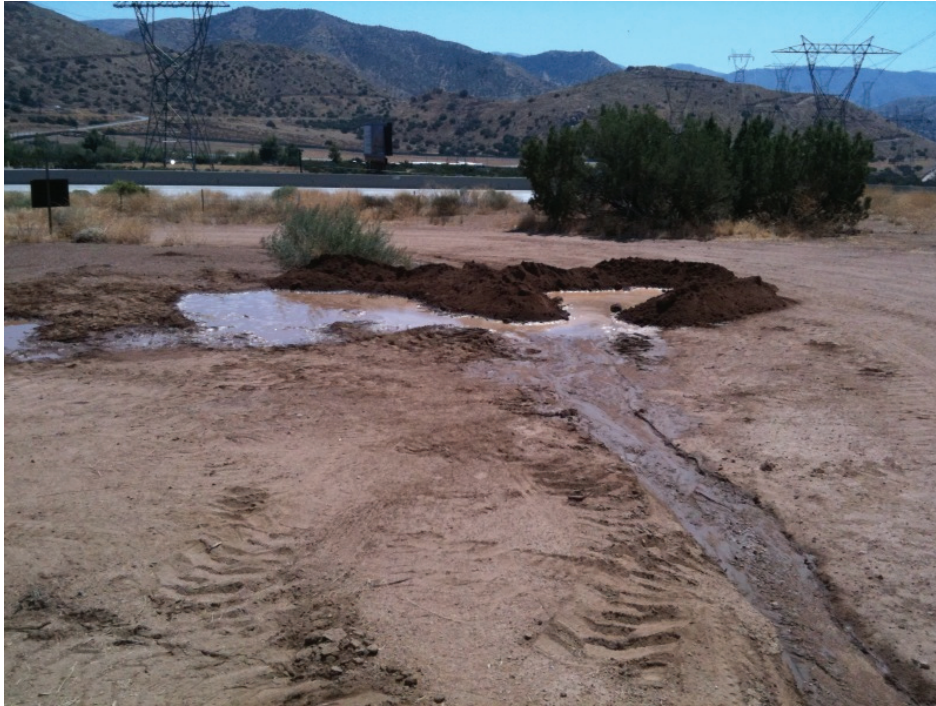
Figure 1: Ponded storm water that was discharged from the trench near Towers 63 and 64, Segment 5.
