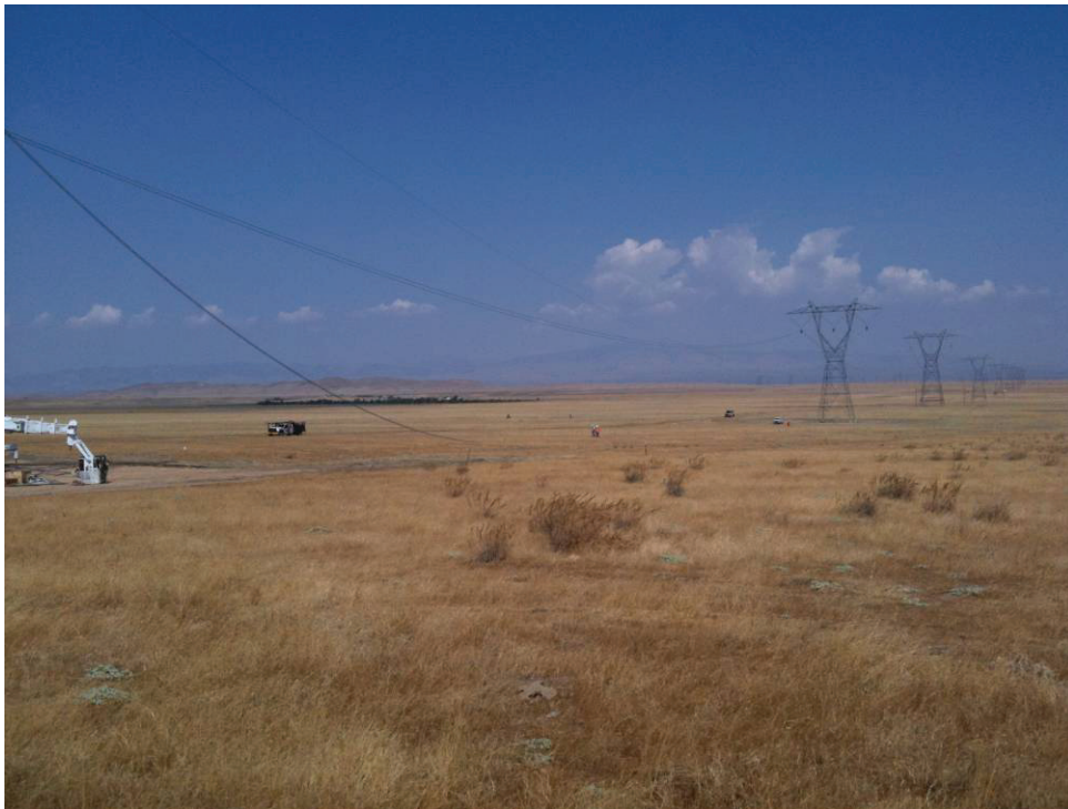
Figure 2: View of conductor touching the ground north of Tower 48, Segment 4.
