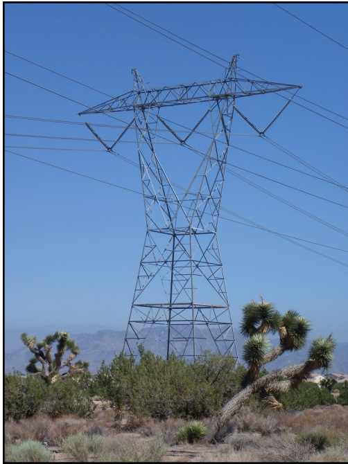
Example of a 500-kV single-circuit LST.
