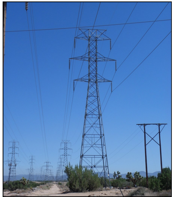
Example of a 220-kV double-circuit LST.
