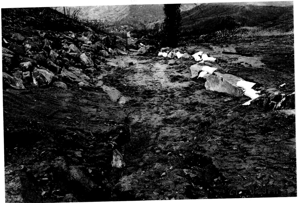
Sandbagged when dirt, river was higher to keep flooding from getting worse!
