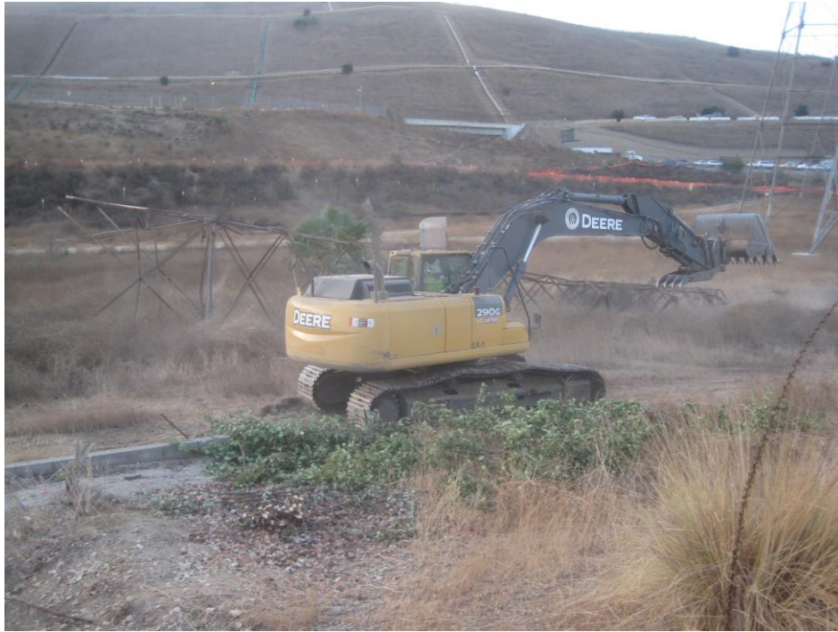
Photo 1: A Power Grade excavator tracking through vegetation in occupied coastal California gnatcatcher habitat on 10/17/2017. The excavator moved a downed lattice tower into vegetation prior to the required pre-construction clearance sweep (Photo by SCE; FRED Incident ID #000021).
