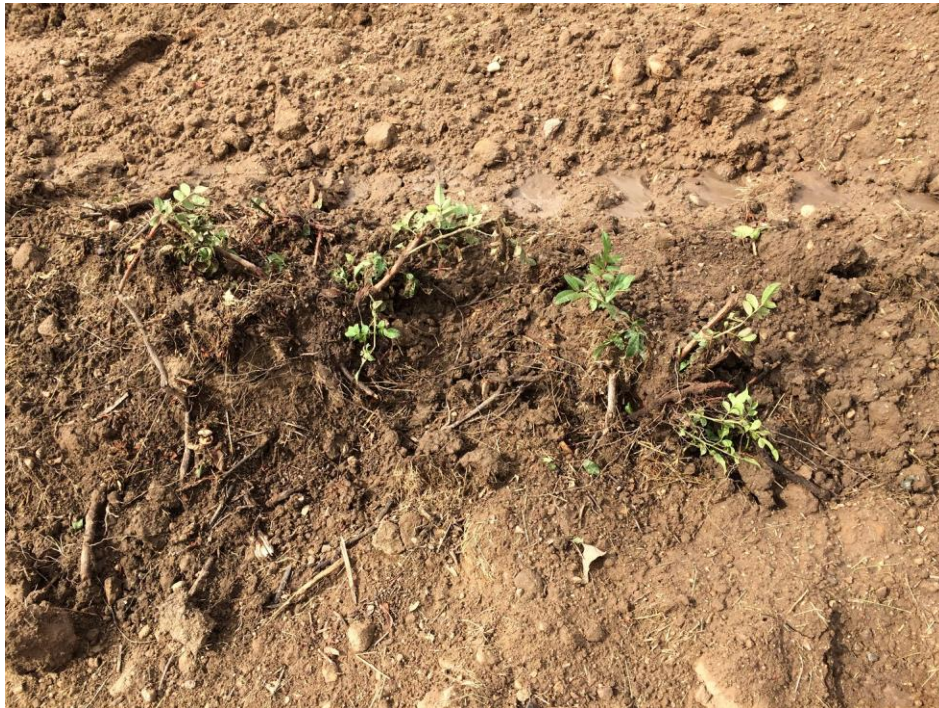
Photo 2: Vegetation removed by a Michels bulldozer on 11/15/2017 in an area that did not have a pre-construction clearance sweep and did not have a biological monitor present (Photo by SCE; FRED Incident ID #000024).
