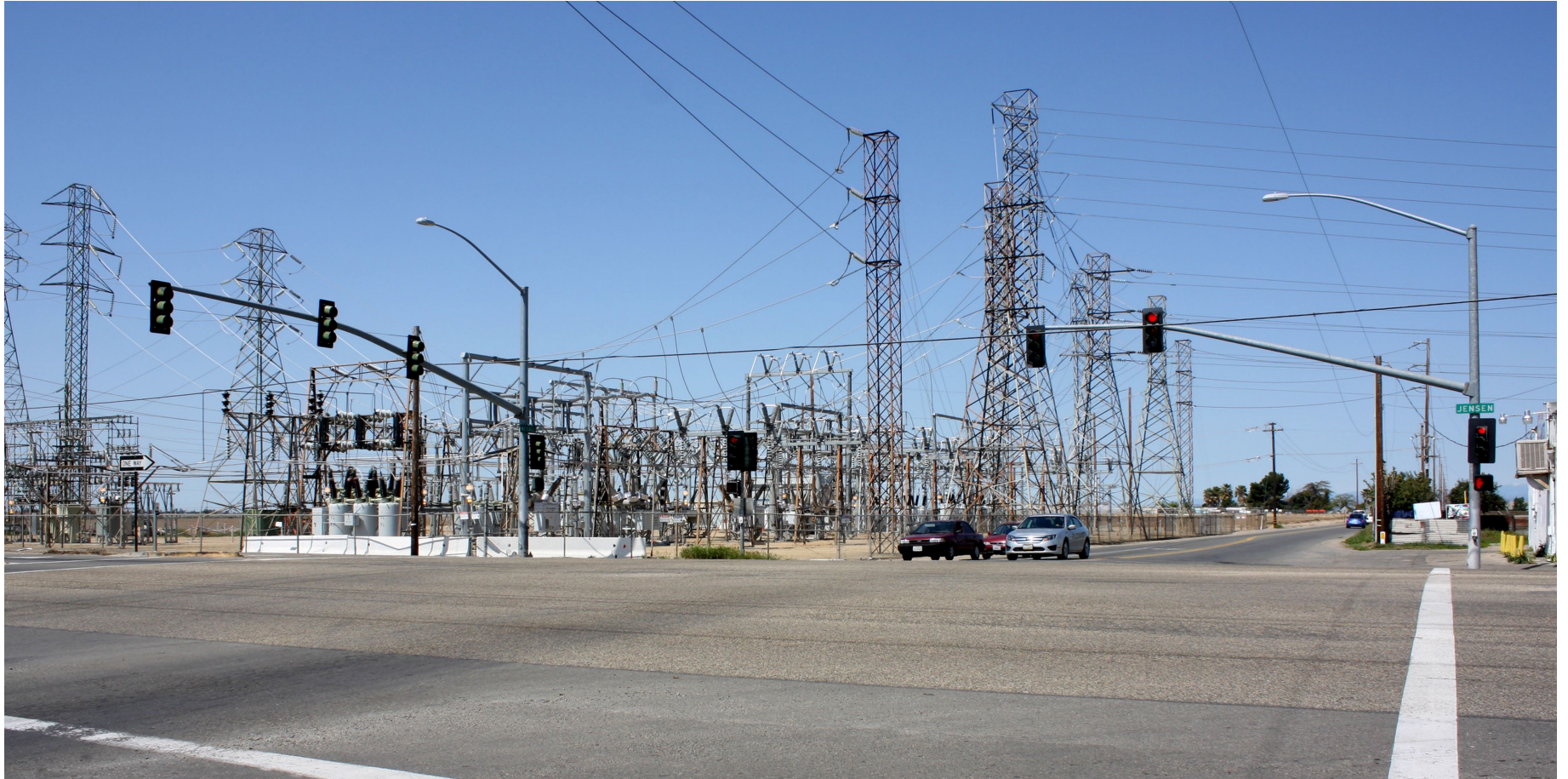
Existing View from South McCall Avenue at East Jensen Avenue looking Northwest (VP 1)
