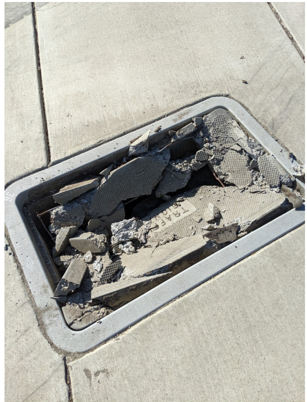
Close up of cracked box cover due to dump truck
