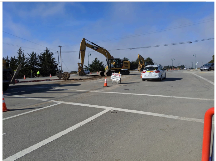
high voltage power line signage as warning for backhoe operators, facing NW
