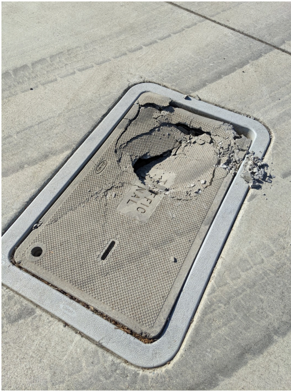
Close up of box cover due to dump truck
