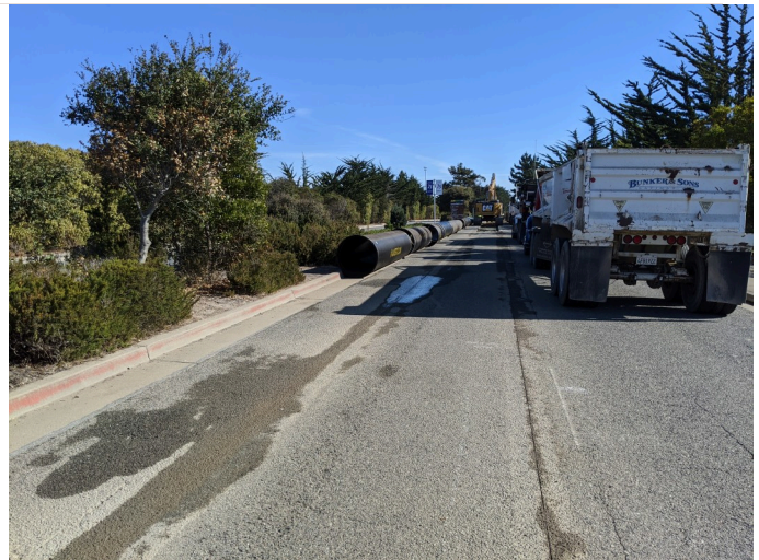
staging of pipeline in roadway in approved work area on Lightfighter, facing E
