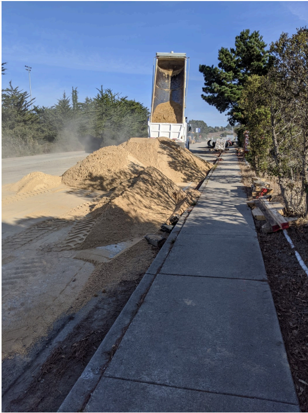
temporary soil storage on site within roadway, on Gen Jim Moore facing N
