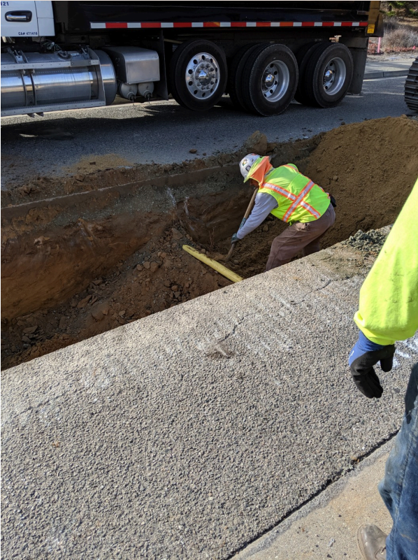
unmarked gas line discovered
