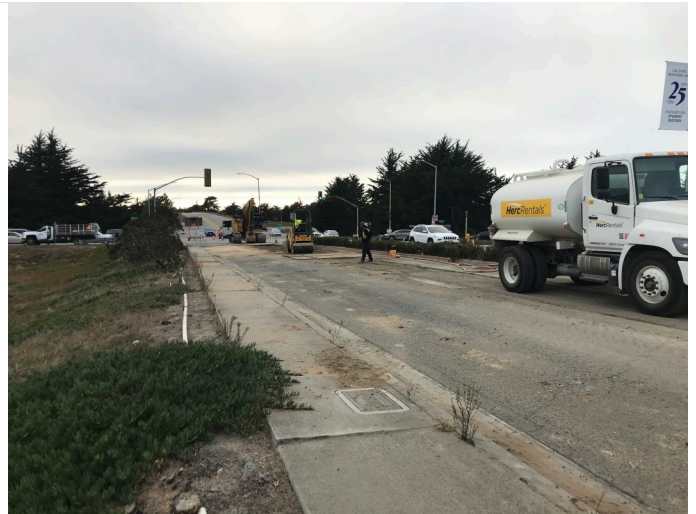
compaction and plates being installed near intersection of First and Light Fighter
