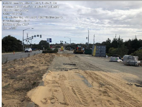
Photo 2. Location of blow off valve on Lightfighter Drive
