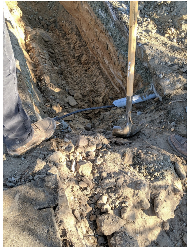
Power line discovered parallel to Lightfighter. Valve trench crossed the line at STA 25+27
