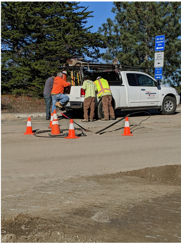
Sudden Link came to repair the disturbed telecom line that was discovered
