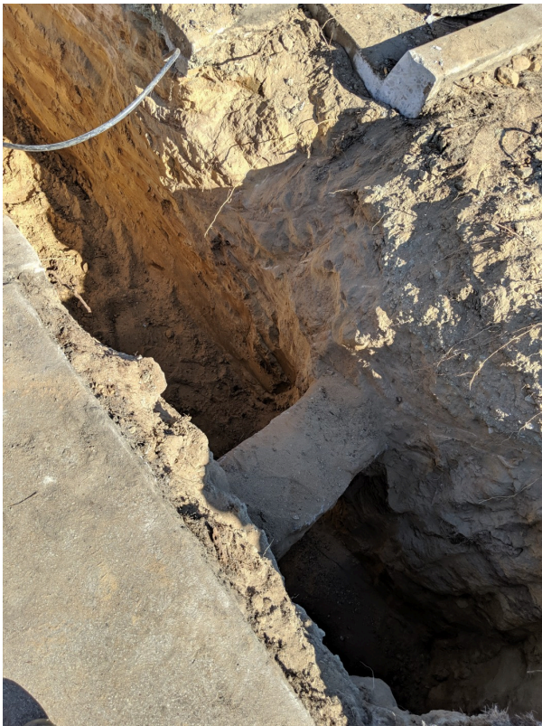
Concrete covered power line discovered parallel to Lightfighter. Valve trench crossed the line at STA 25+27
