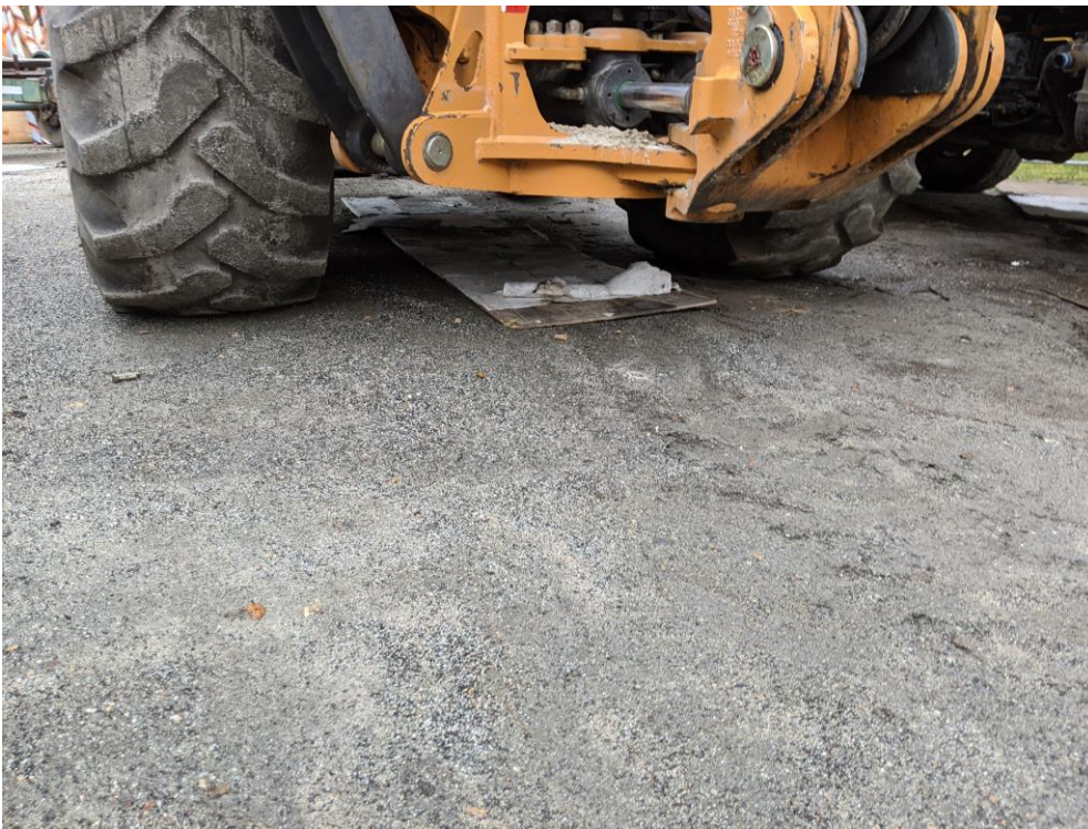
Photo 4. Hazardous spill protection under parked equipment in staging area. (3-30-2020)
