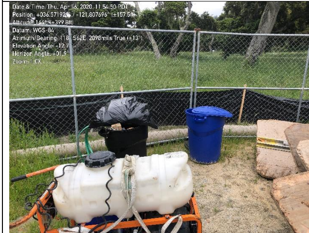
Photo 3. Trash receptacles not properly contained within staging area.
