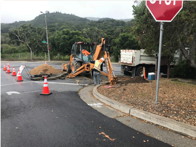
installation of air valve at the corner of York Rd and Wilson Rd
