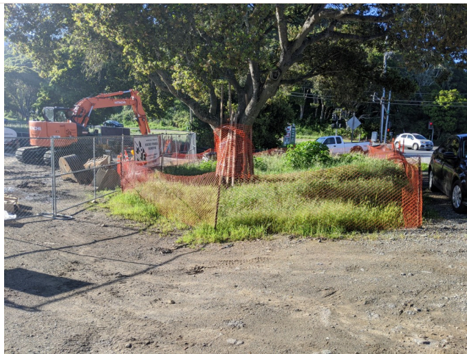
View of intact esa fencing around protected oak tree adjacent to staging area
