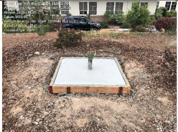
Photo 2. Installed ARV components.
