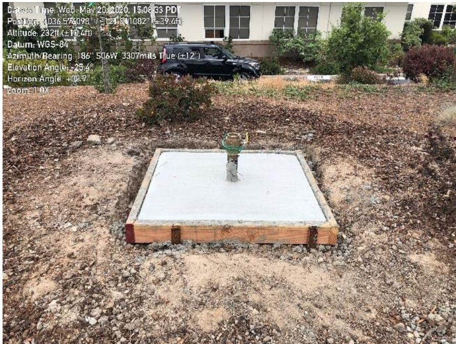
Photo 2. Installed ARV components.
