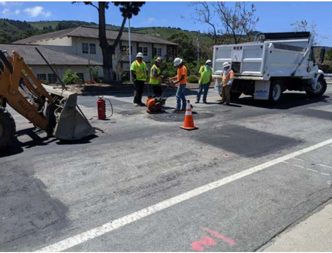
MPE paving over ARV valve collars along alignment on Lower Ragsdale Drive.
