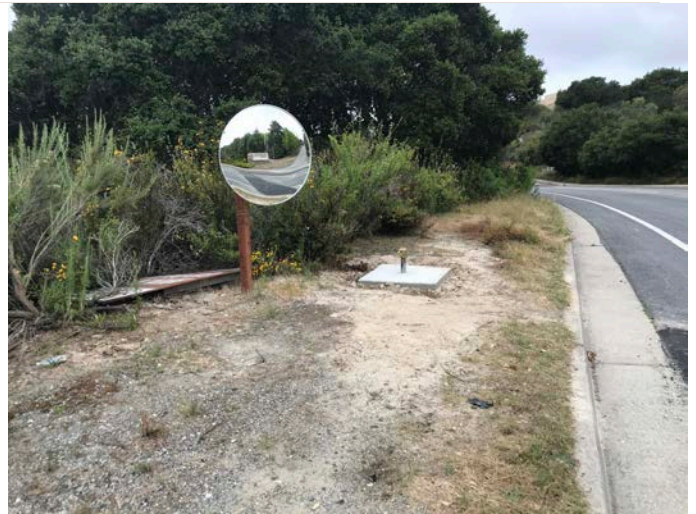
Recently installed pad for the Air Release Valve along Lower Ragsdale Rd
