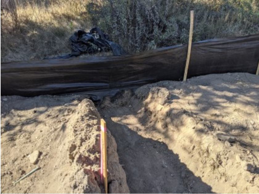
10/27/2020 - Section of compromised exclusionary fencing, notified crew.
