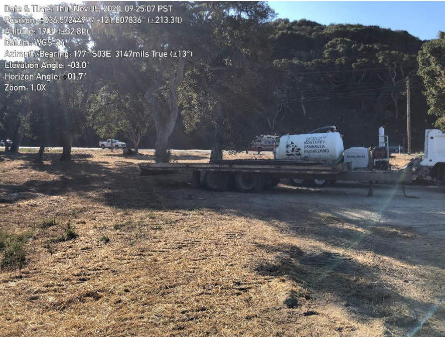
Photo 6. Ryan Ranch – Bishop Interconnection Improvements: Equipment parked outside of staging area limits.
