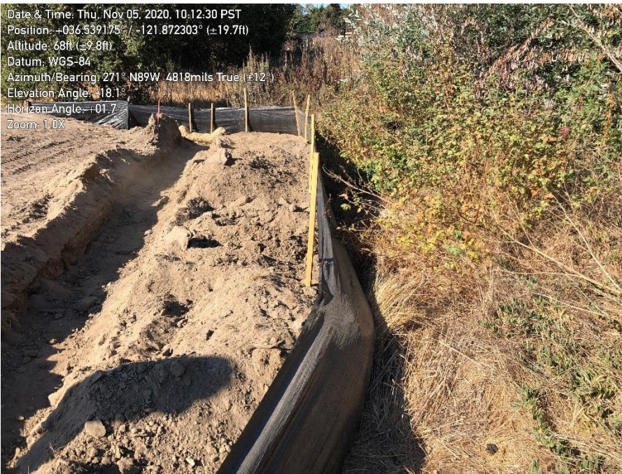
Photo 2. Carmel Valley Pump Station: small section of silt fence compromised.
