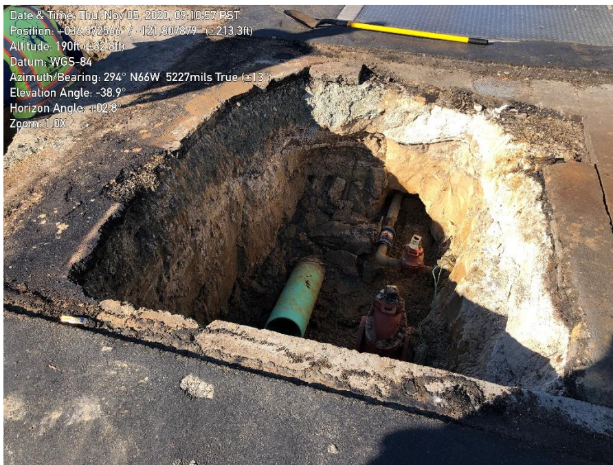
Photo 4. Ryan Ranch – Bishop Interconnection Improvements: Installation of tie-in on Blue Larkspur Lane.
