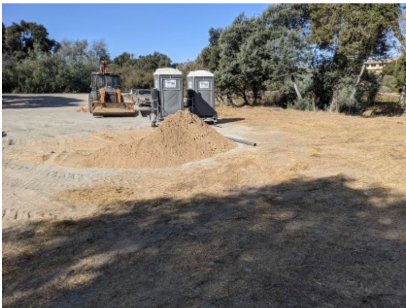
11/05/2020 - Equipment/vehicles parked within unapproved staging area.
