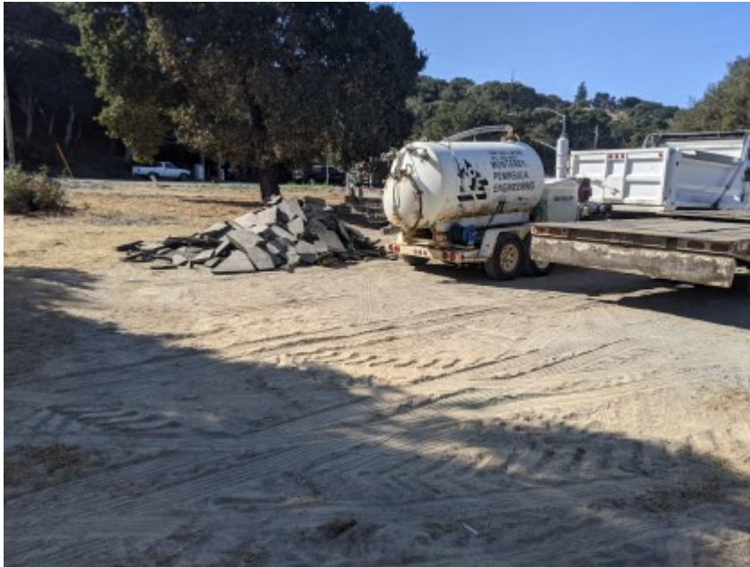
11/05/2020 - Equipment/vehicles parked within unapproved staging area (Roadbase confirmed removed as of 11/6).
