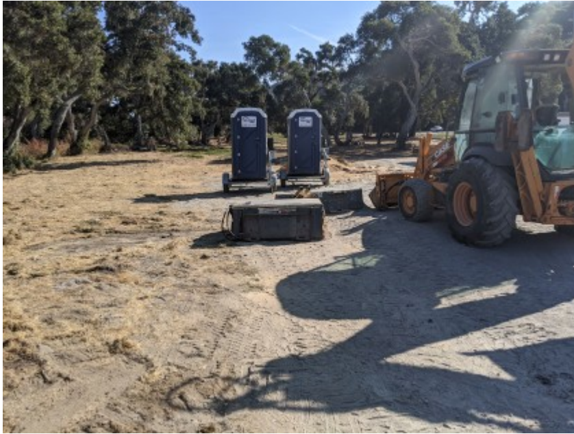
11/05/2020 - Equipment/vehicles parked within unapproved staging area.
