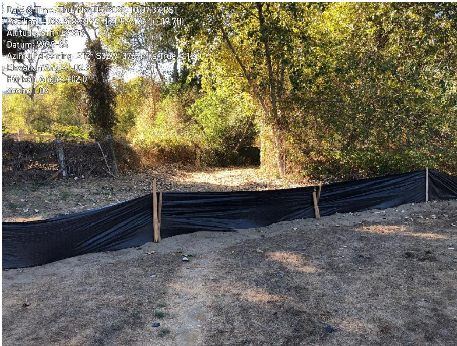
Photo 1. Carmel Valley Pump Station: newly installed silt fence to exclude additional parking/staging area.
