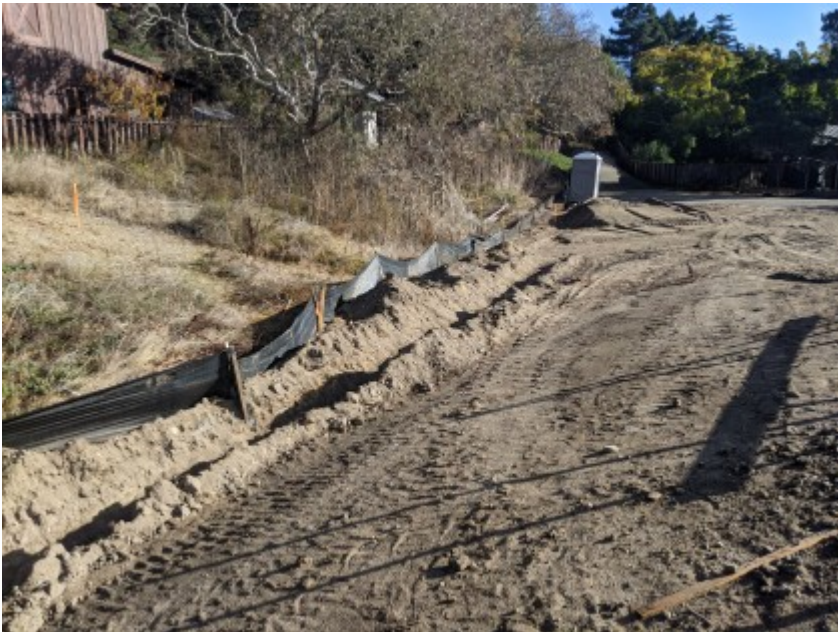
11/16/2020 - Soil building up against silt fencing in need of removal
