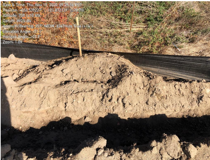
Photo 1. Carmel Valley Pump Station: small section of silt fence compromised.
