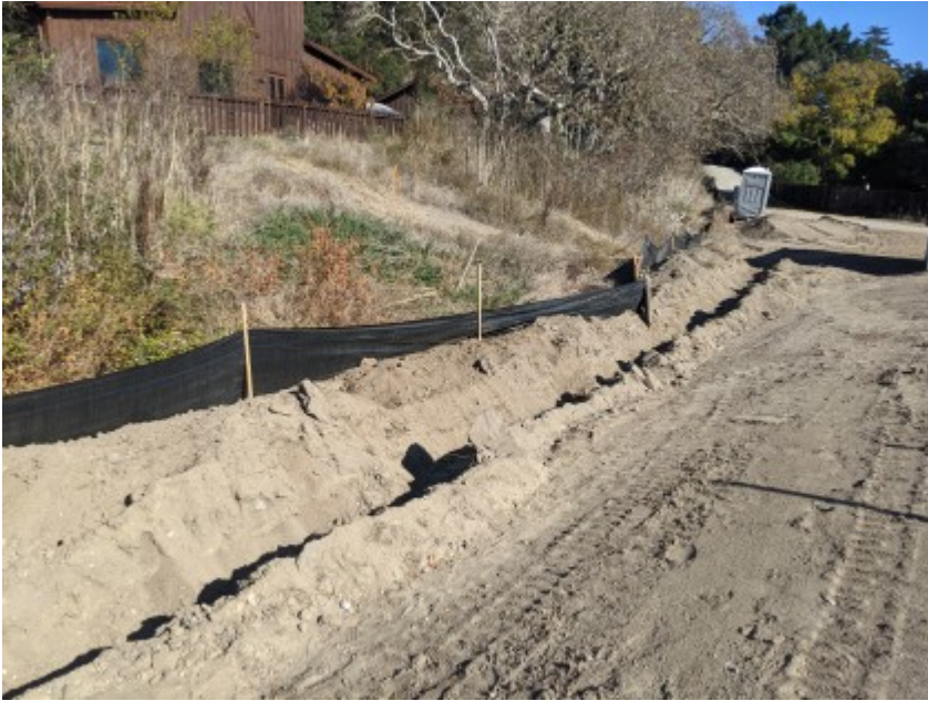
11/24/2020 - Soil building up against silt fence removed.
