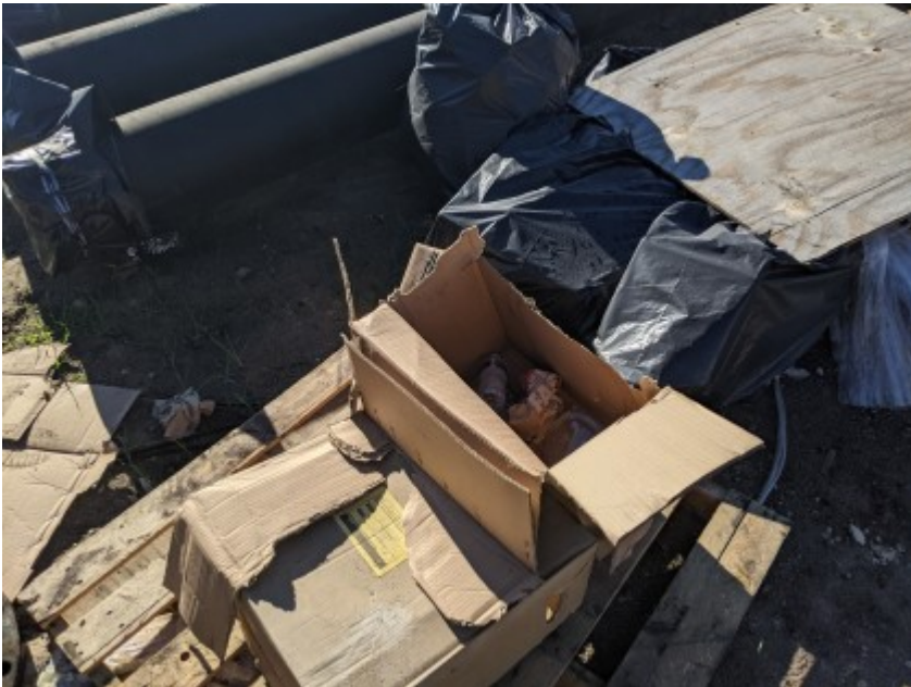
01/14/2021 - Improper disposal of food/trash scraps within work area.
