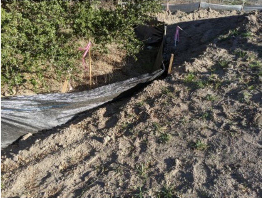
01/21/2021 - Section of exclusionary fencing being covered by eroded soil from work area in need of repair.
