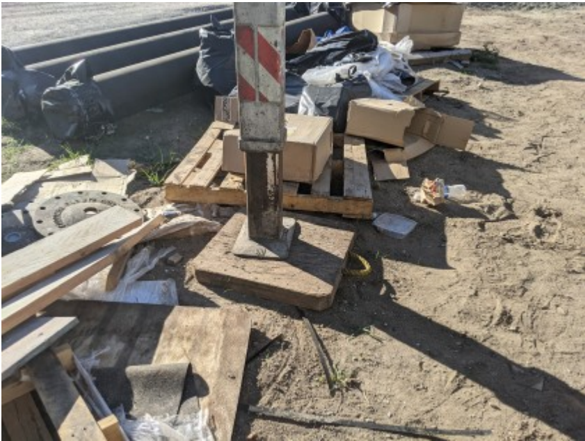
01/21/2021 - Food/trash scraps within work area in need of cleanup.
