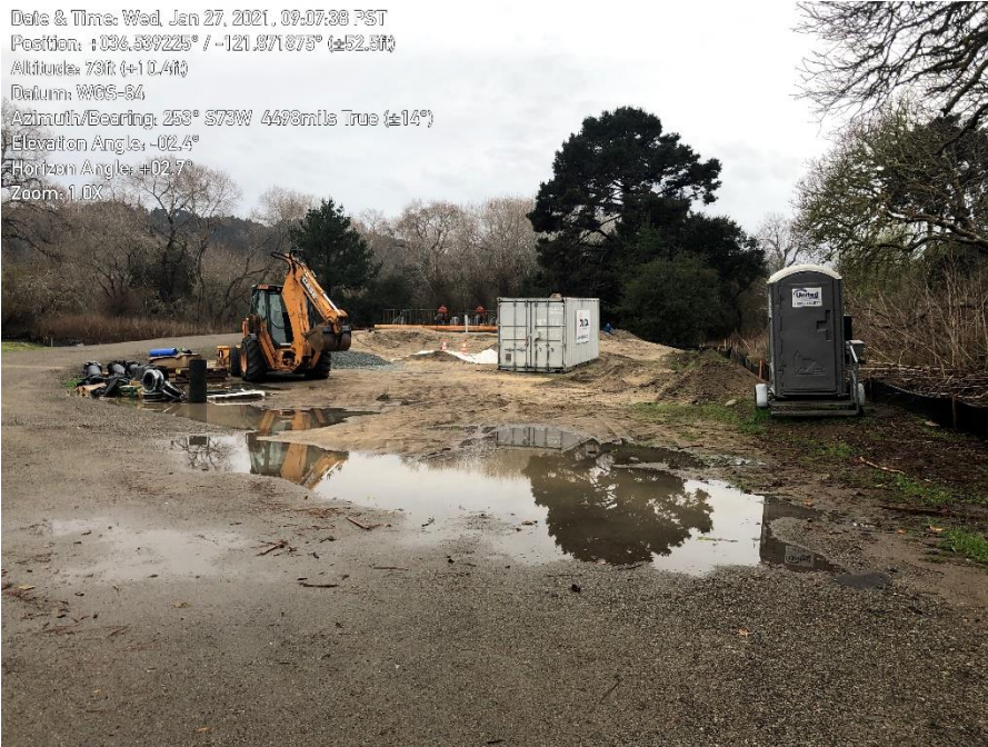
Photo 1. Site conditions after rain event.
