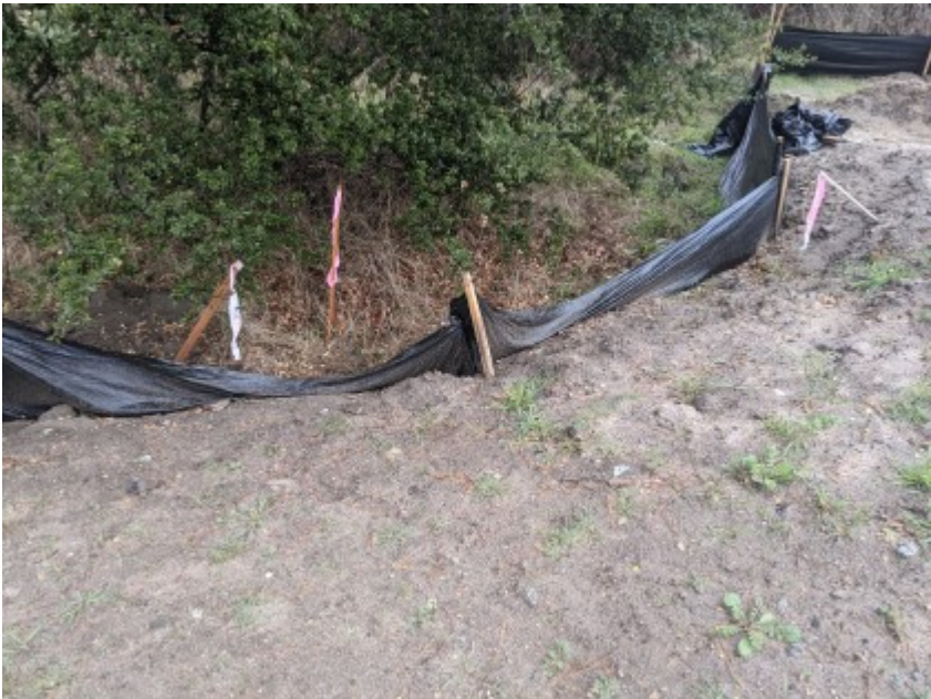
01/27/2021 - Erosion within work area damaging exclusionary fencing.
