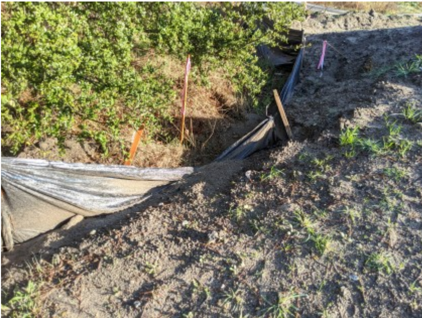
01/29/2021 - Erosion within work area damaging exclusionary fencing.
