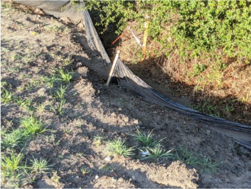
01/29/2021 - Erosion within work area damaging exclusionary fencing.
