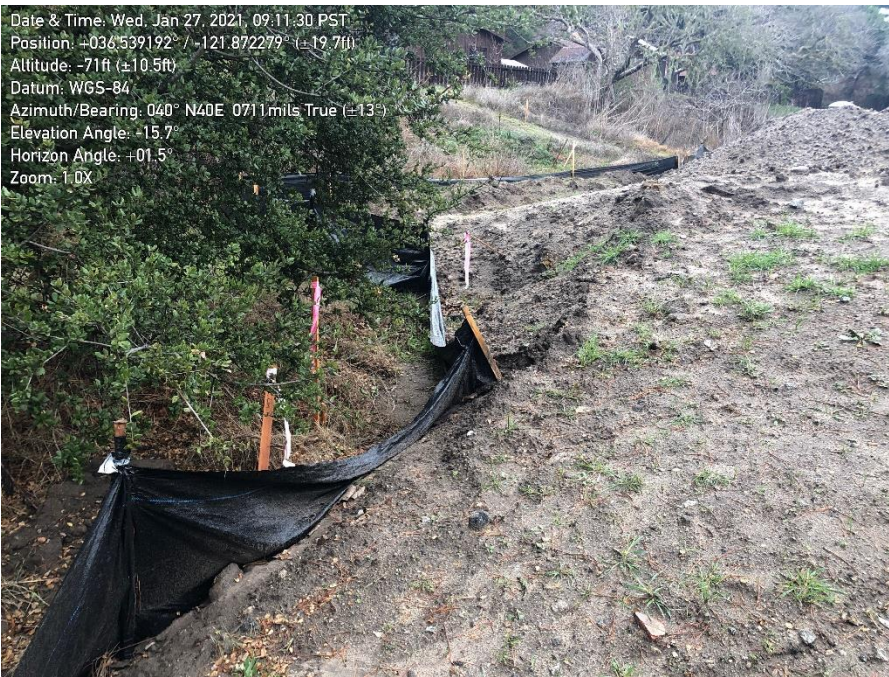
Photo 5. Silt fence down and in need of repair.
