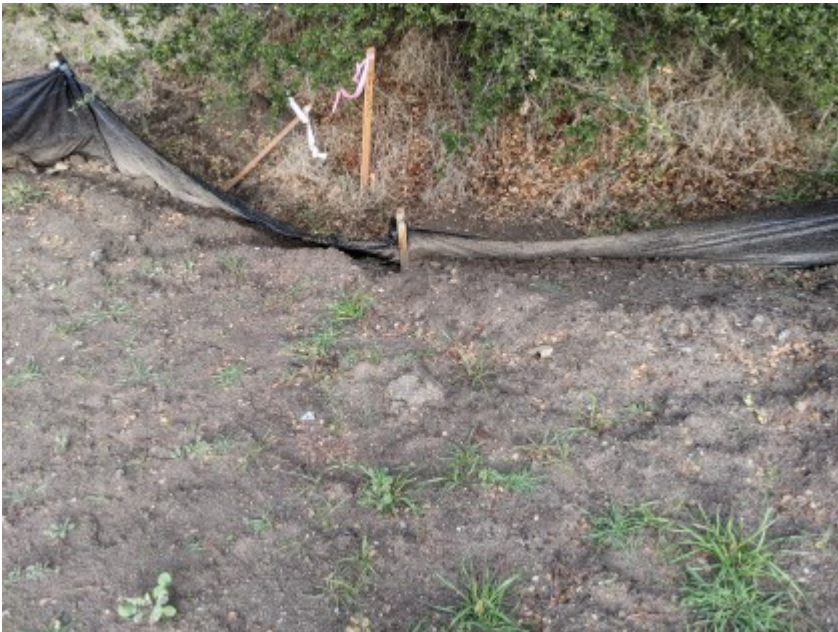
01/25/2021 - Erosion within work area beginning to damage exclusionary fencing.
