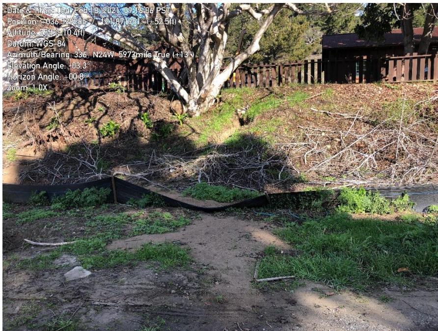
Photo 2. Silt fence compromised due to erosion.
