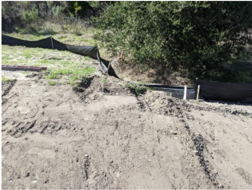
02/18/2021 - Section of exclusionary fencing damaged by erosional feature.
