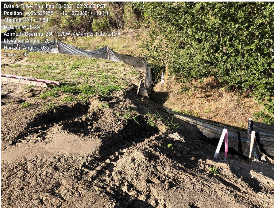
Photo 4. Silt fence down and in need of repair.
