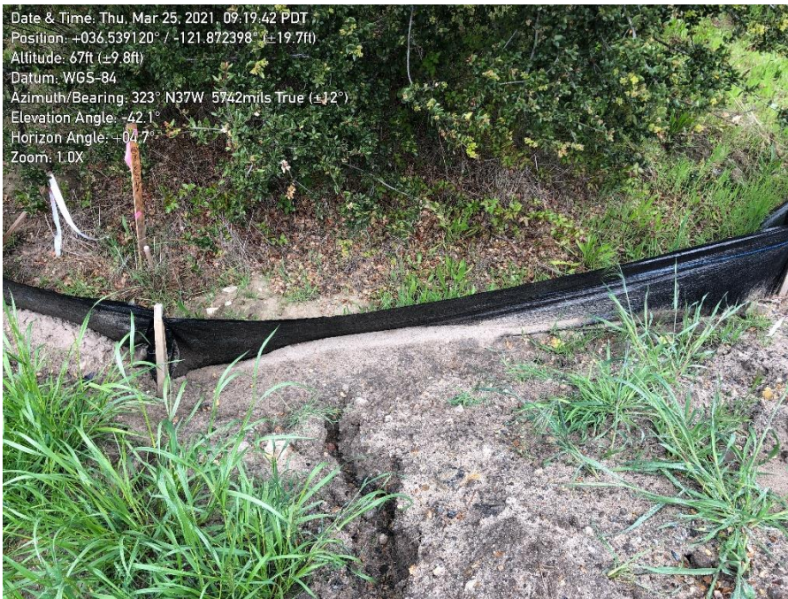
Photo 5. Sediment backed up along silt fence near pad.
