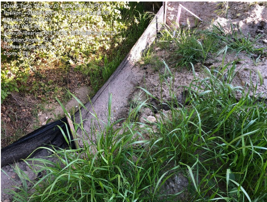
Photo 4. Sediment backed up along silt fence near pad.
