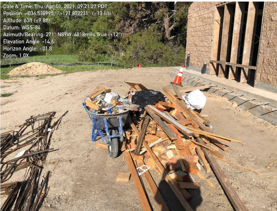
Photo 6. Trash improperly disposed of in wheelbarrow.
