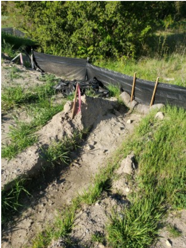
04/01/2021 - Drainage feature installed on northern boundary of project site.
