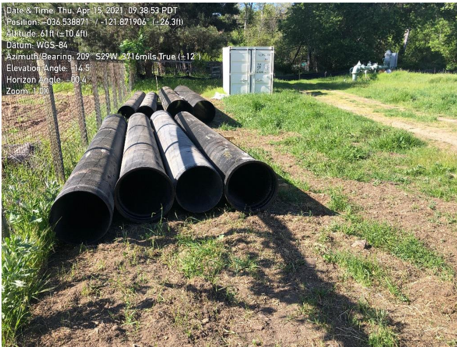
Photo 3. Uncapped pipes should be inspected prior to moving.
