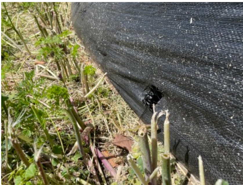
04/16/2021 - Holes caused by vegetation removal are still in silt fence, need to be fixed.
