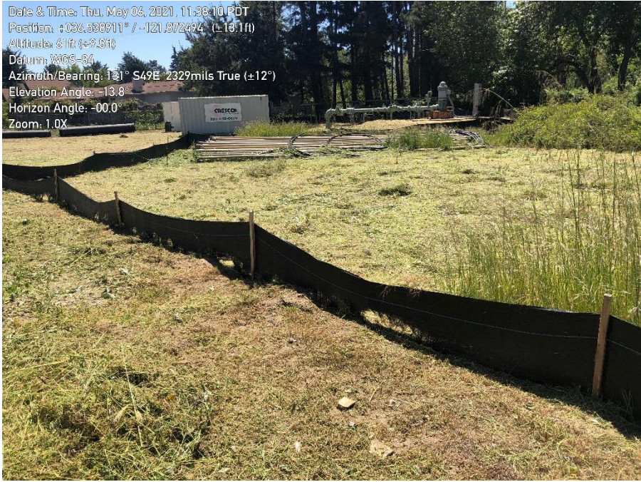
Photo 1. Mechanical weeding activities inside and outside of exclusion fence. Exclusion fence has been damaged by weed removal activities.
