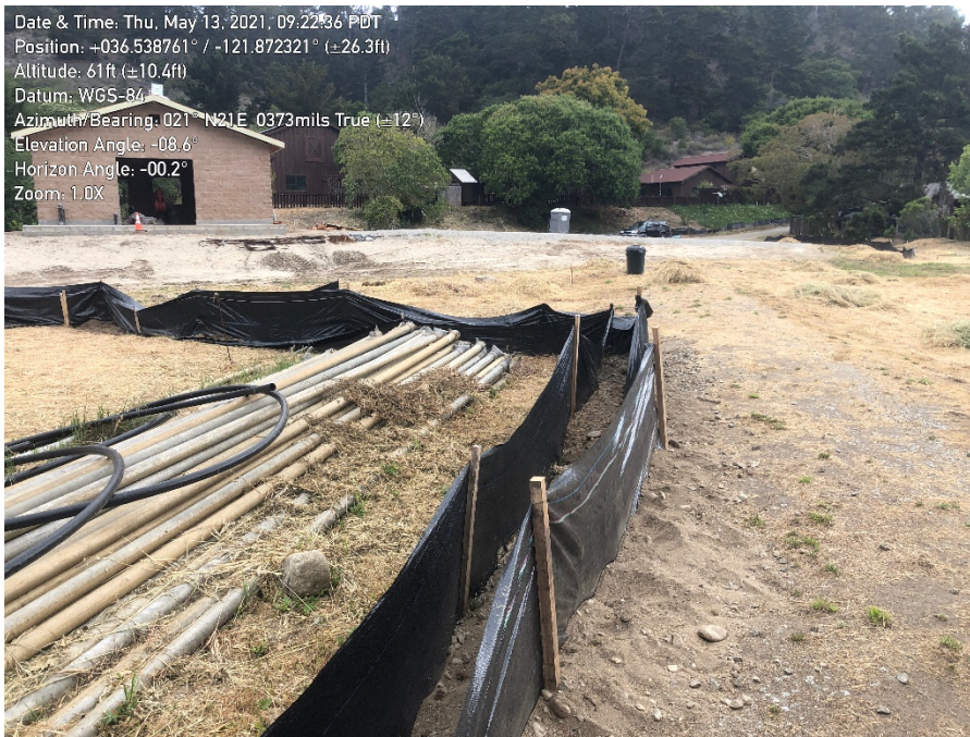
Photo 3. New silt fence installed adjacent to damaged silt fence.
