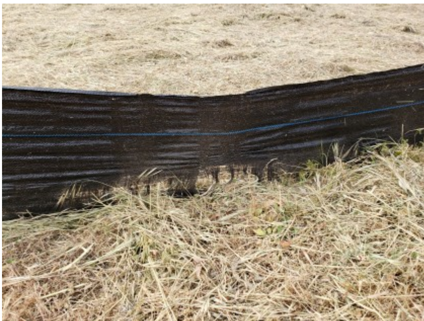
05/13/2021 - Exclusion fencing to be repaired.
