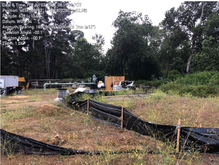
Photo 2. Portion of exclusion fence not keyed in. Fence repaired during site inspection.
