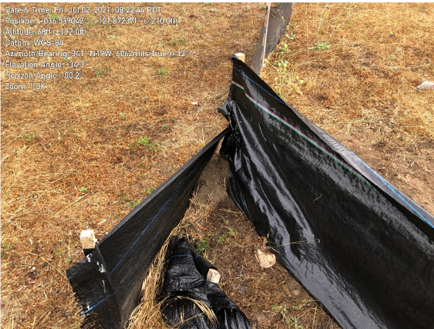
Photo 1. Gap in fence.
