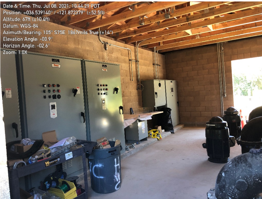
Photo 1. Pump station interior.
