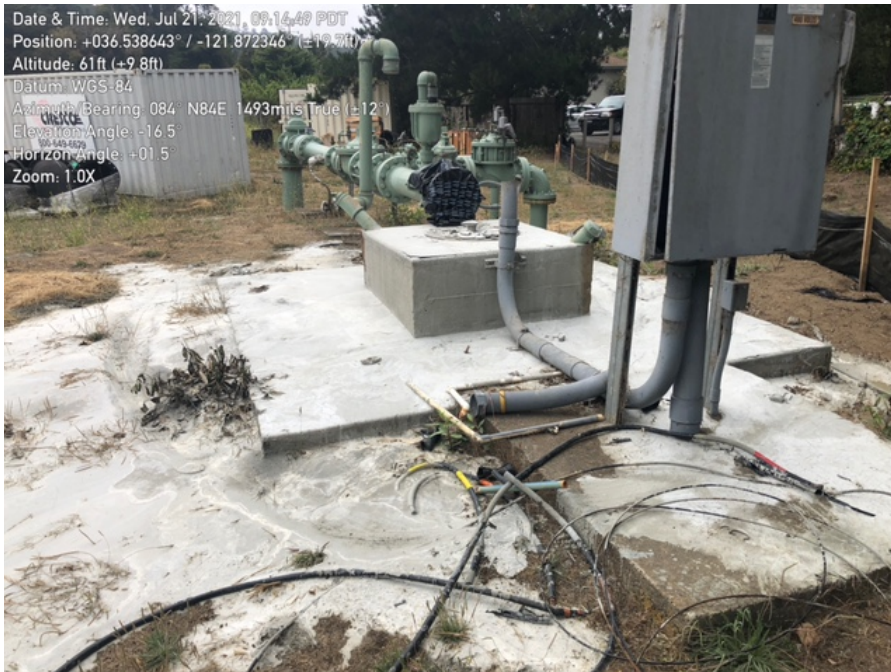
Photo 4. Old well has been filled with concrete. Pipe capped to prevent wildlife entry.
