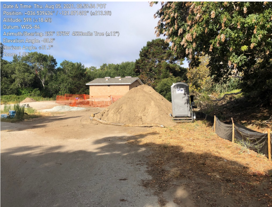
Photo 1. Site conditions. Monofilament wattle observed around stock pile.
