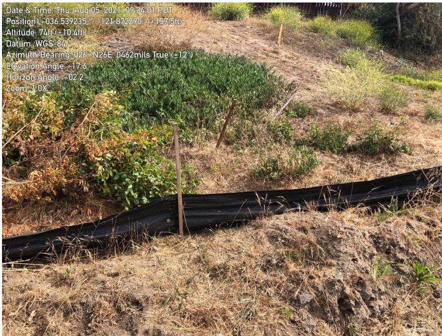
Photo 3. Silt fence in need of repair along north border.
