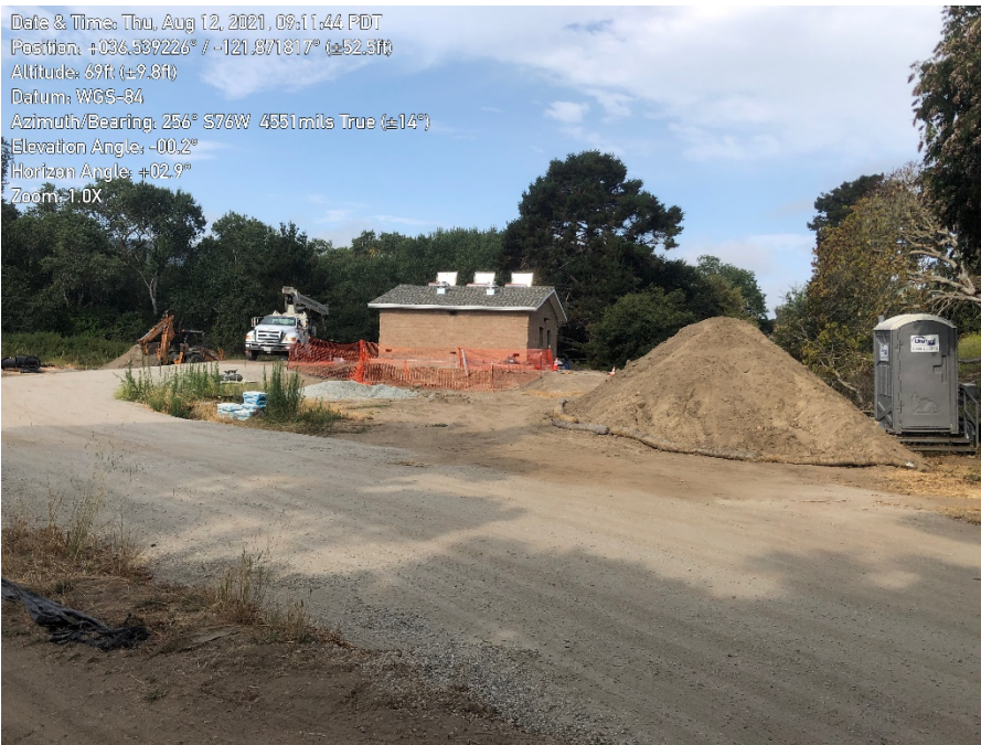
Photo 1. Site conditions. Monofilament wattle observed around stock pile.
