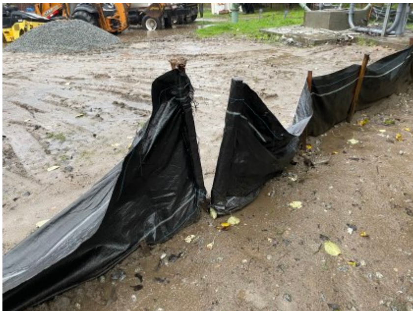
12/14/2021 - Downed silt fencing that needs to be repaired. Repaired by DD&A on 12/16/2021.
