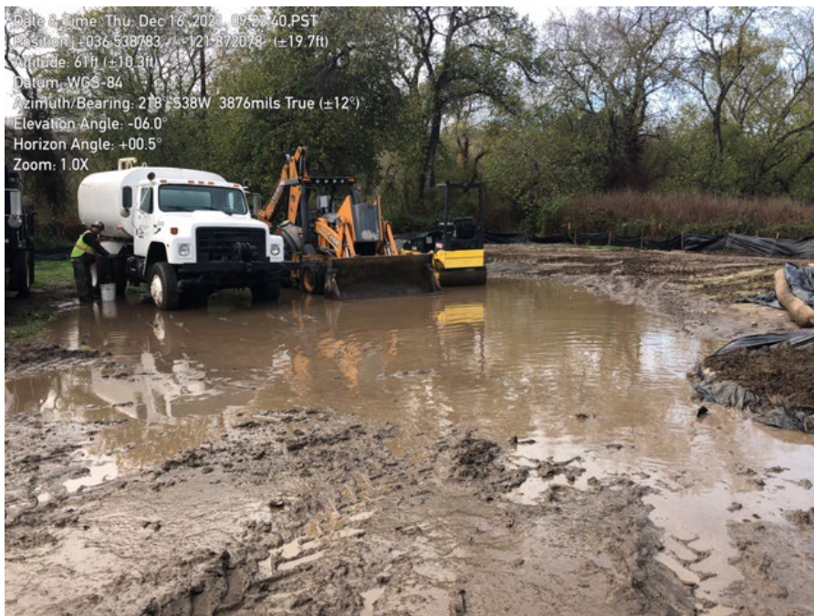
Photo 4. Ponding from recent rain events.
