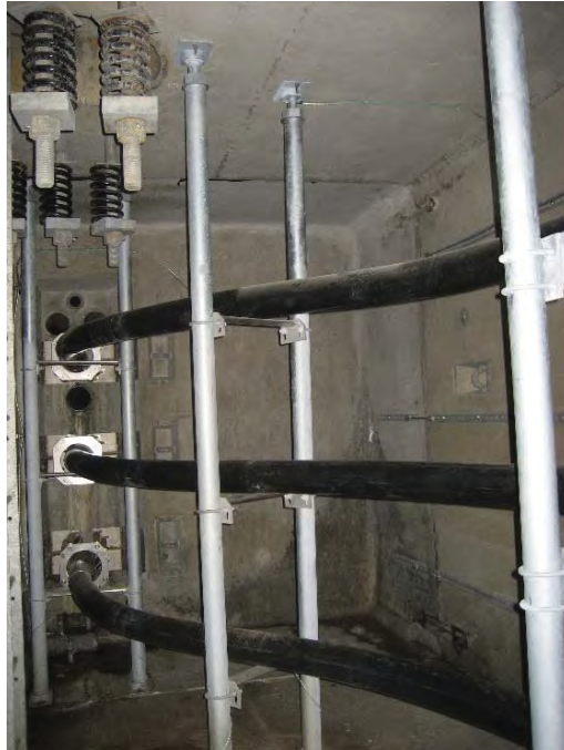
Figure 13: Inside LADWP 230 kV Vault
