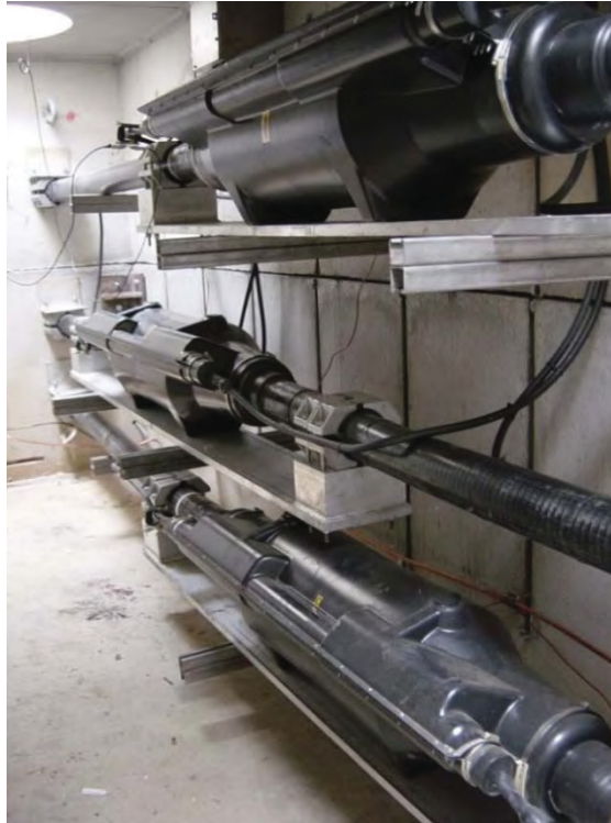
Figure 14: Example of a Completed 230 kV Splice
