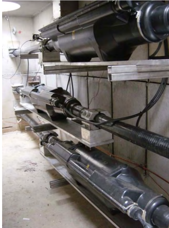
Figure 14: Example of a Completed 230 kV Splice
