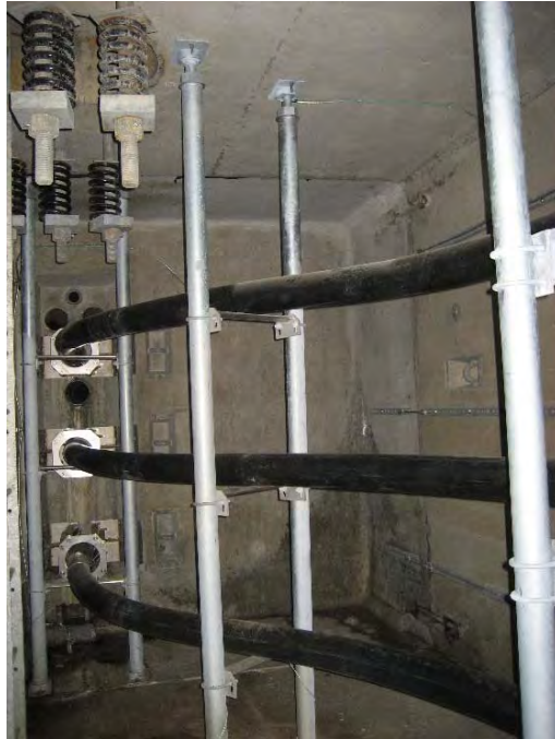
Figure 13: Inside LADWP 230 kV Vault
