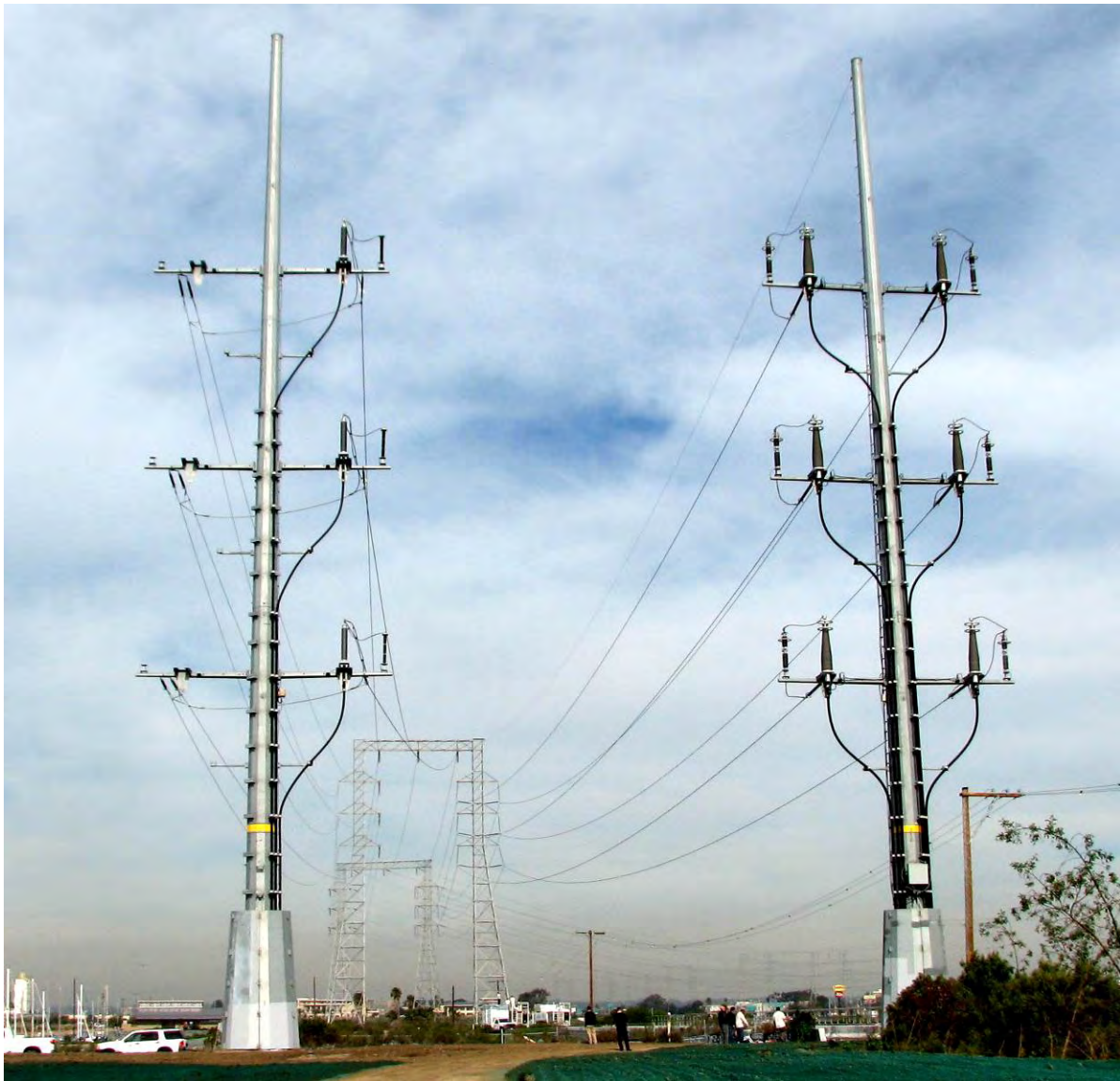
Figure 7: SDG&E Transmission Riser Poles (165 ft. tall and spaced approximately 90 ft. apart)
