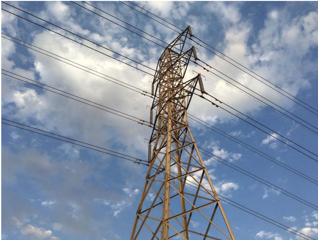
Views from underneath the transmission line at the corona noise measurement location
