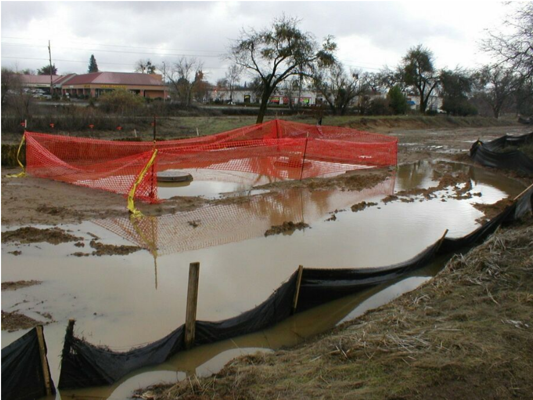
Figure 2 – Standing water near Vault 1 and Wetland 2, December 23, 2005.
