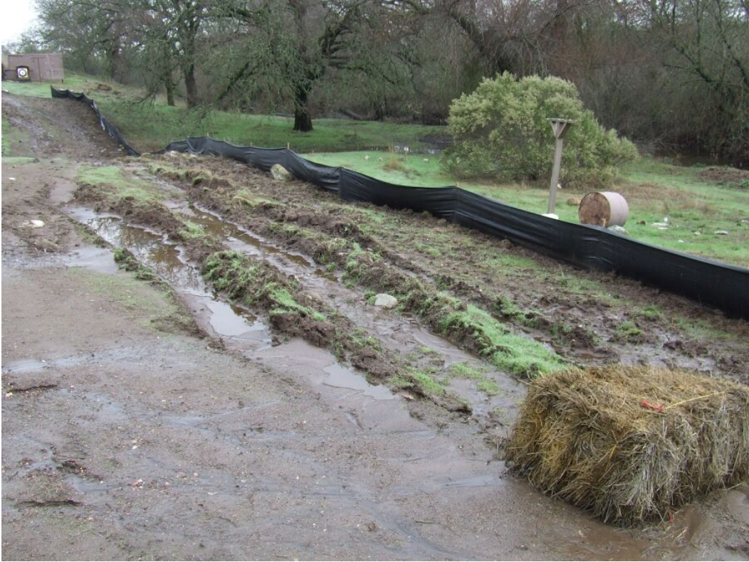
Figure 1 – Rutted access road and erosion control measures, December 29, 2005.
