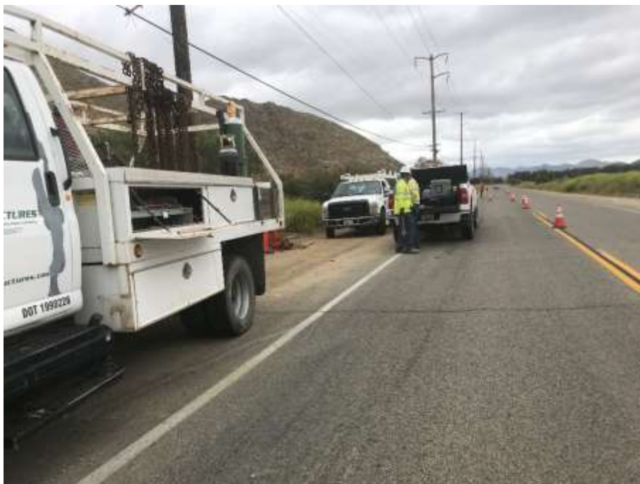
Photo 2 – Traffic control along Matthews Road during foundation drilling activities at Construction Area UNK 02, May 7, 2019.
