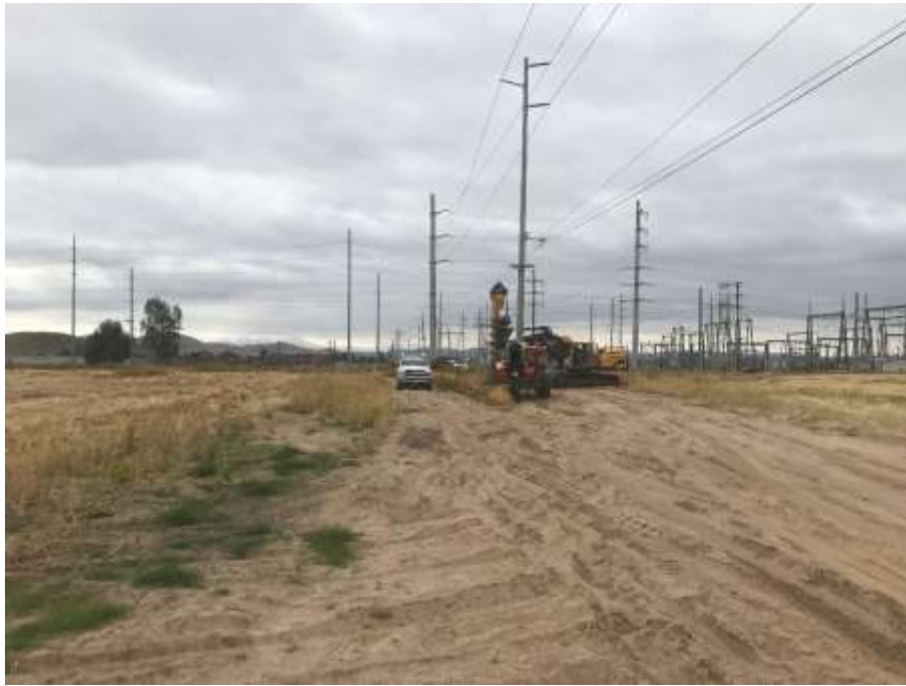
Photo 1 – Foundation drilling took place outside of the Valley Substation at Construction Area UNK 250, May 7, 2019.
