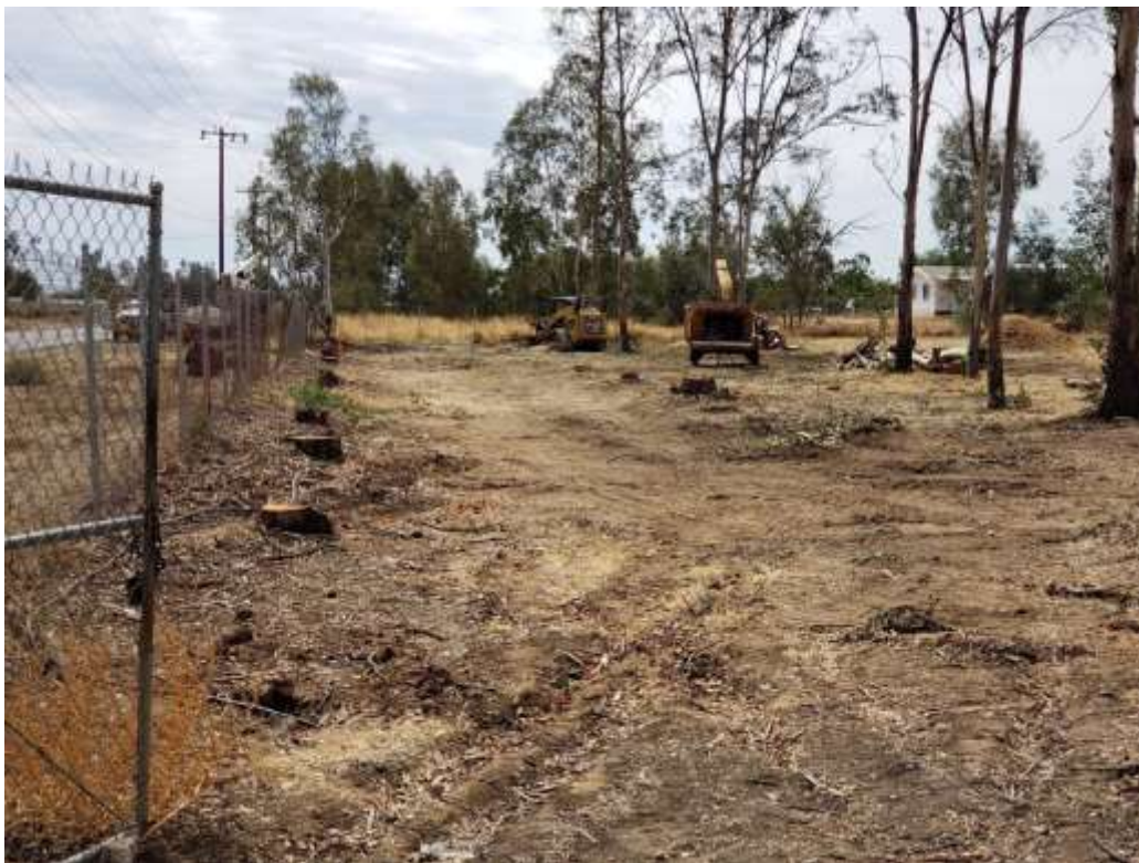
Photo 4 - Tree trimming and vegetation clearing at Construction Areas UNK177 and UNK178 (September 25, 2019).
