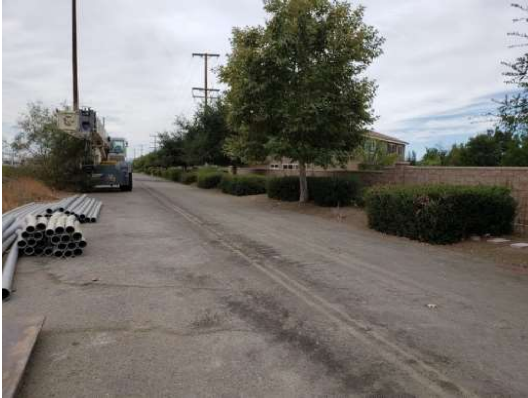
Photo 5 – Uncapped pipes and a piece of construction equipment staged without secondary containment near UNK222 (September 25, 2019).
