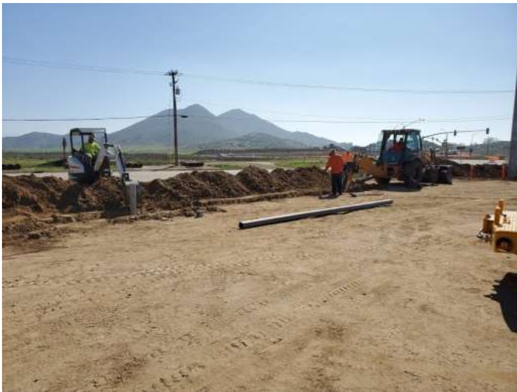
Photo 4 – Trenching outside approved project disturbance area limits between Construction Areas UNK44 and UNK45 (February 19, 2020).
