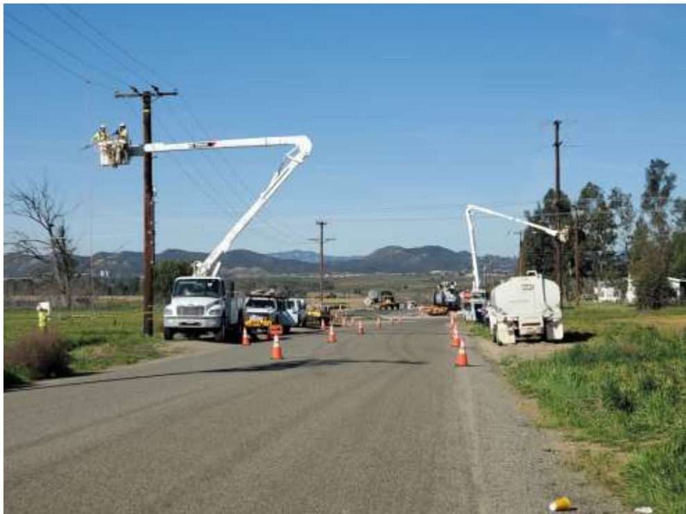
Photo 2 – Distribution reconductoring and wreck-out at Construction Area UNK180 and pole 4163134E (March 4, 2020).
