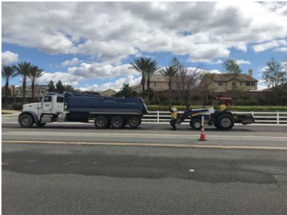
Photo 2 – Paving of Leon Road at Construction Areas UNK207 through UNK222 (March 24, 2020) (Photo courtesy of SCE).
