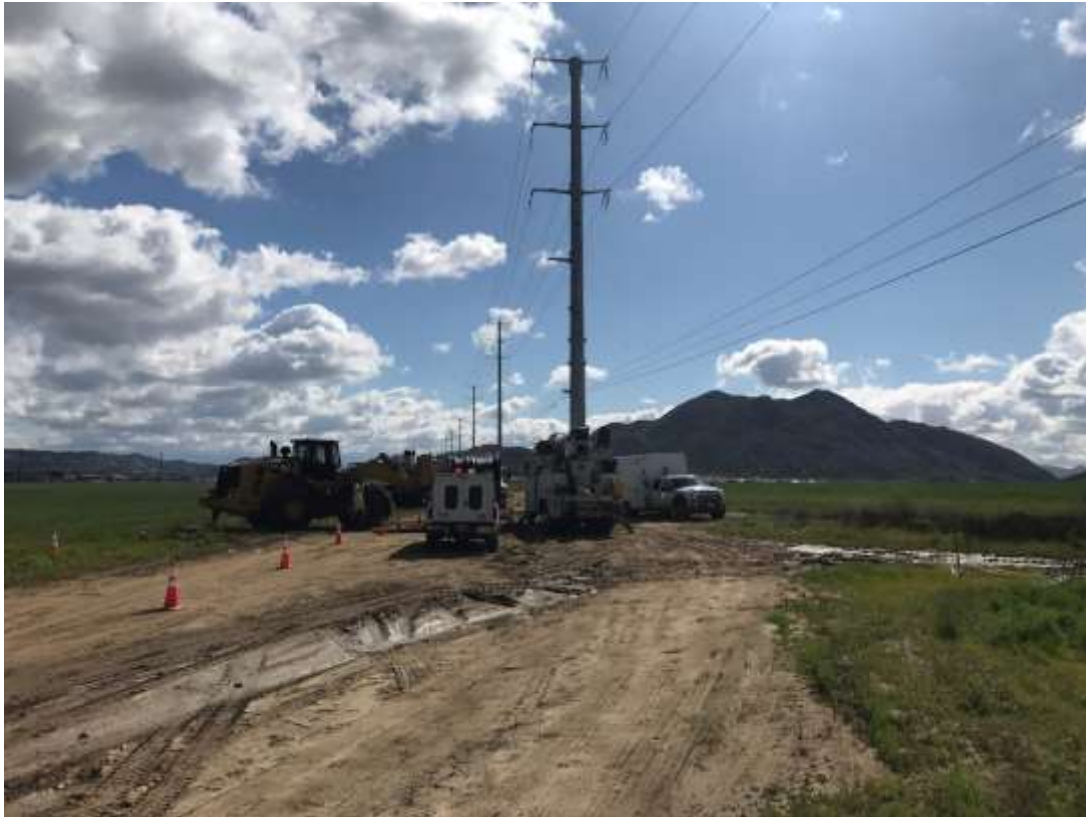
Photo 3 – Pulling cable at the underground vault at Construction Area UNK250 (March 26, 2020) (Photo courtesy of SCE).
