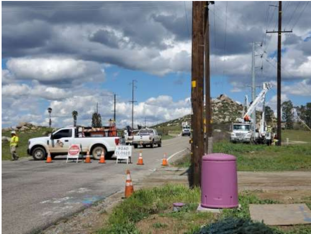
Photo 1 – 115 kV subtransmission wire stringing activities at Construction Area UNK125 with traffic control on Leon Road (March 17, 2020).
