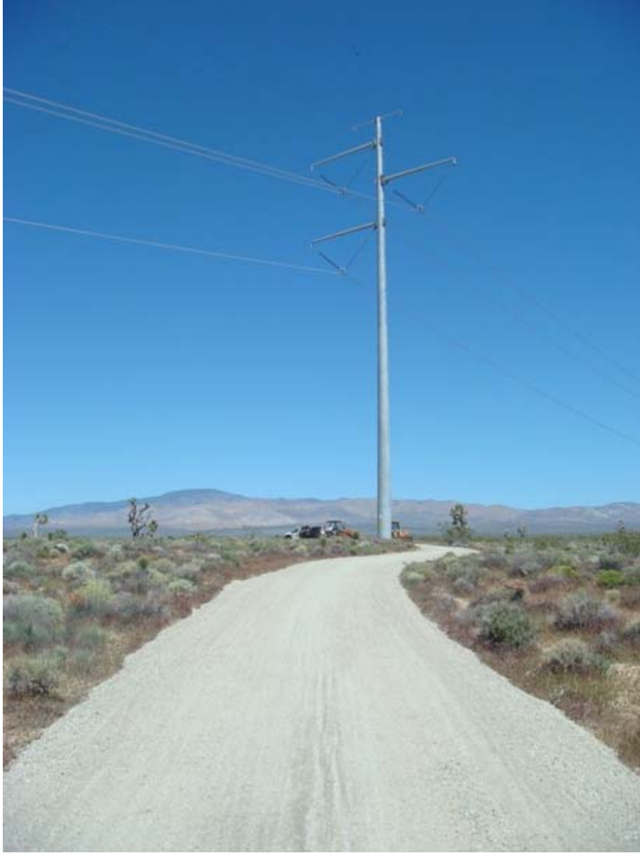
Figure 1: Road capping was completed to provide Operation and Maintenance access to Tower 43 in Segment 3A.
