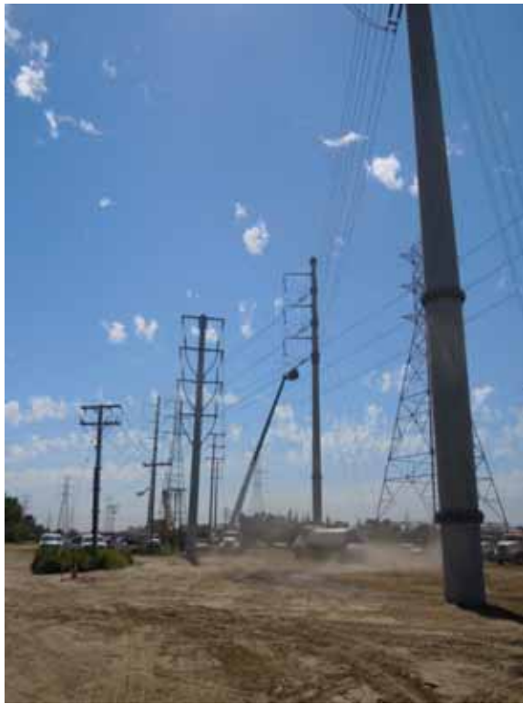
Figure 7: Crews string a shoofly pole near I-605 as a water truck sprays water underneath, Segment 8 Phase 4.
