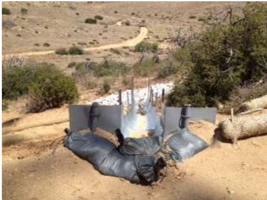
Figure 2: Metal storm drain at Construct 51A, Segment 5.
