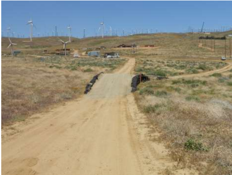
Figure 1: Gravel cover to protect an existing pipeline that crosses the access road between Structures 31 and 32, Segment 3B.
