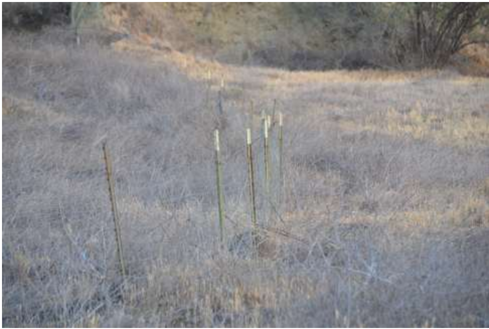
Figure 3: Remnants of silt fencing in the Haskell Canyon area from Segment 1.
