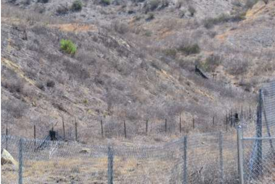
Figure 1: Silt fencing installed surrounding a dirt stockpile area in Segment 1 in non-functioning condition.
