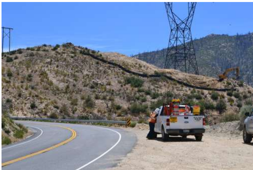
Figure 5: Grading at Construct 23 with construction traffic flaggers along Angeles Crest Highway, Segment 6A.
