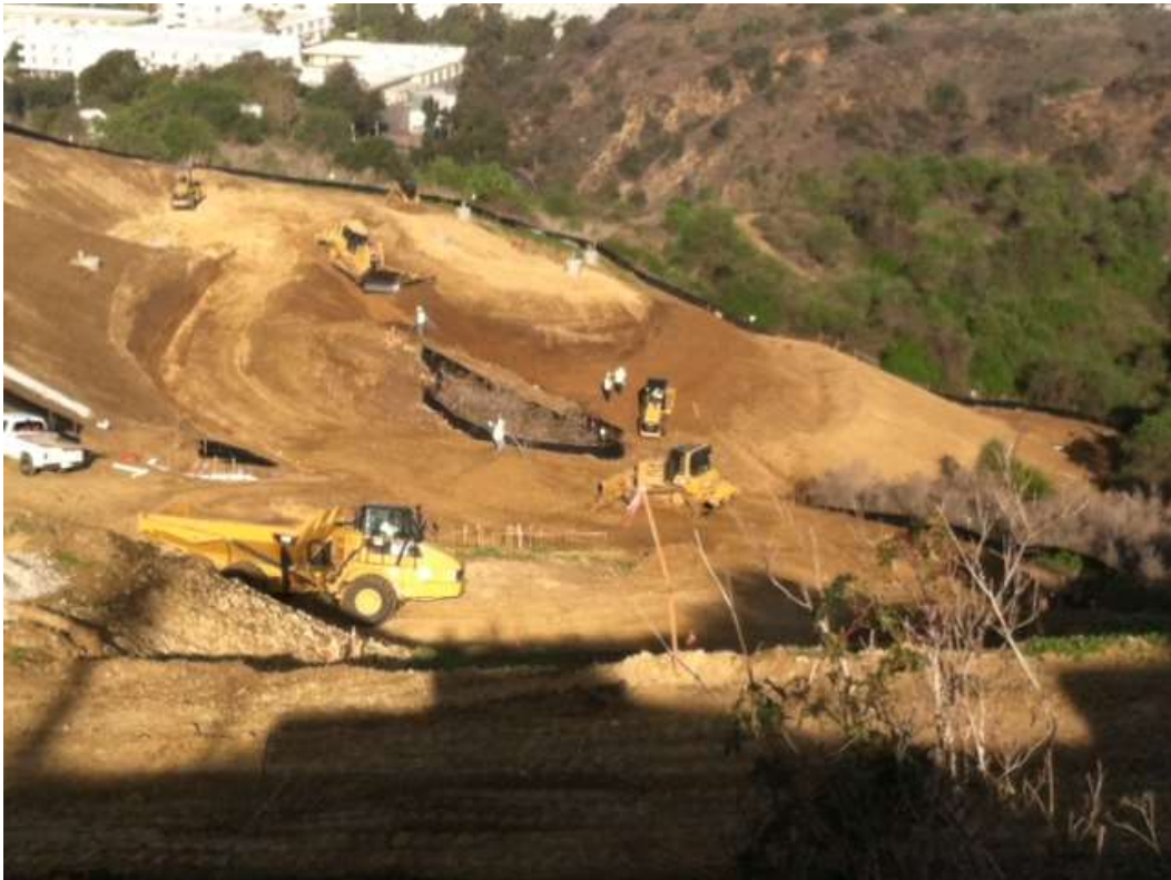
Figure 7: Patriot Construction crews grading access road and tower site at M43-T3, Segment 8.
