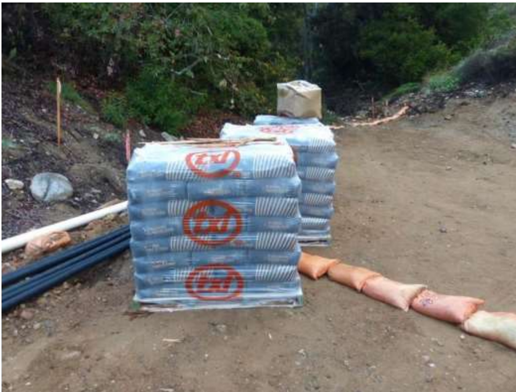
Figure 8: Materials stockpiled within an Environmentally Sensitive Area (jurisdictional drainage) during a rain event at Tower M27-T3, Segment 7. Photo courtesy of FRED.
