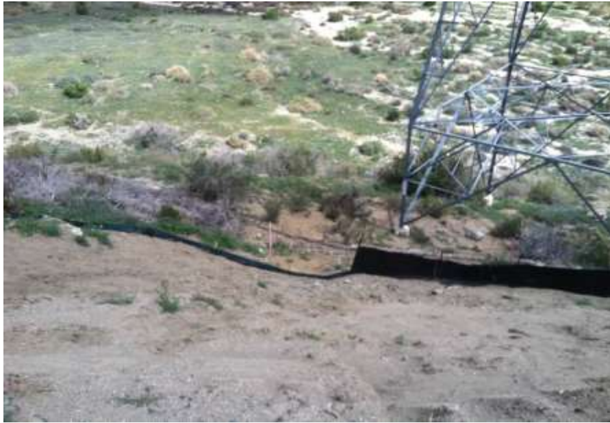
Figure 1: Erosion control devices were installed at the outstanding locations identified in the CPUC NCR, Segment 6, Tower 10. Although these devices were installed, additional work to clean up offsite erosion is still needed.
