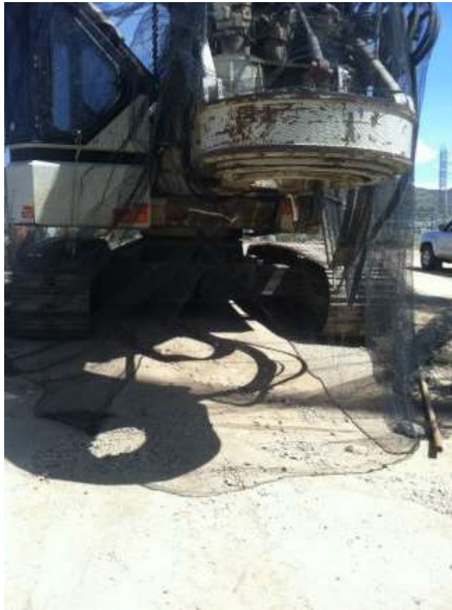
Figure 3: Bird deterrent netting draped over a crane with large gaps, SCE was notified of the concern.
