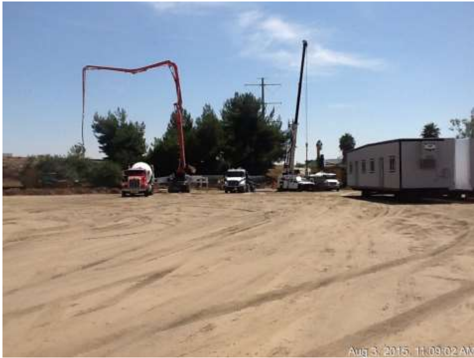
Figure 3: Concrete pour for the transition tower foundation at the ETS, 500 kV Underground.
