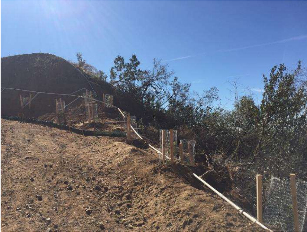
Figure 1: Container plant installation at Tower M27-T3 on Segment 7.
