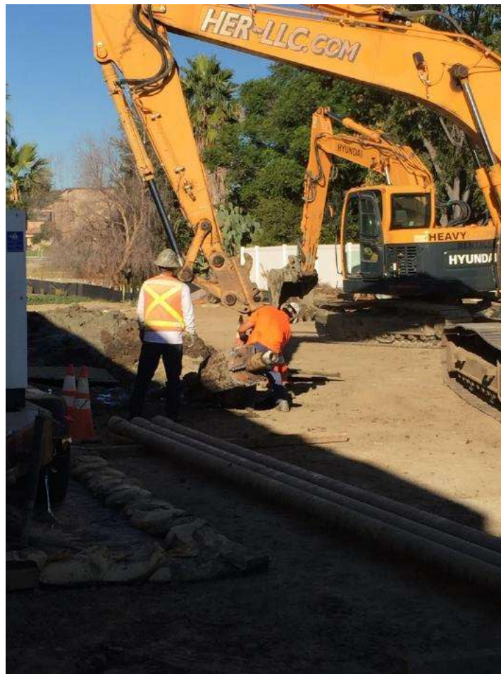
Figure 4: HDD reaming operations continue near VC #12 at the long bore location, 500 kV Underground.
