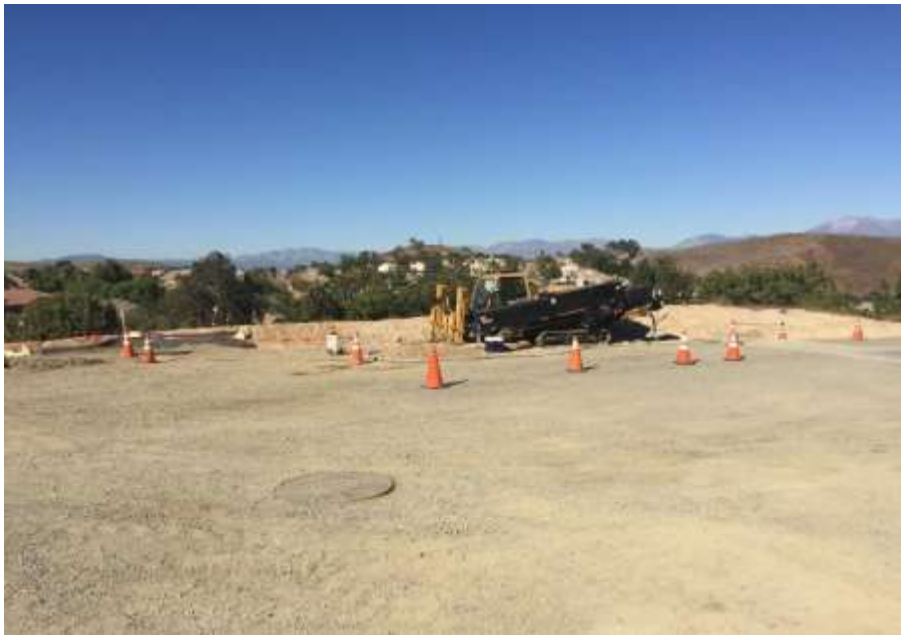
Figure 3: HDD set up near VC #1 to install telecom system into the WTS, 500 kV Underground.
