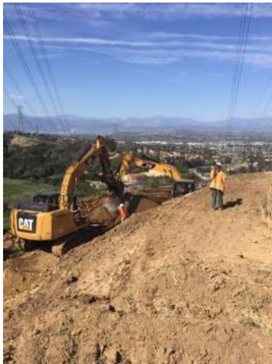
Figure 2: Civil work for slope stabilization is ongoing at Tower MA1-T2A, Segment 8 Phase 4.
