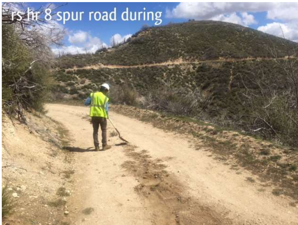
Figure 2: During weed abatement photo of Loop Road O, Segment 11C. Photo courtesy of SCE.
