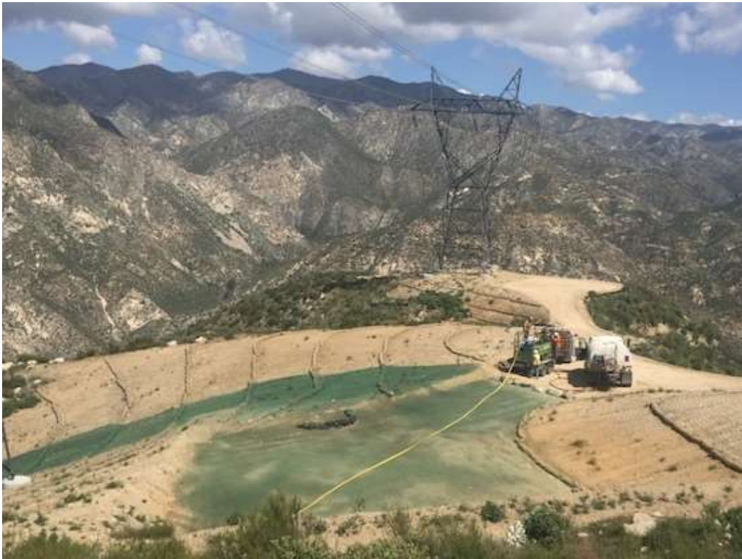
Figure 3: Restoration maintenance (hydroseed application) at Tower 54, Segment 11C. Photo courtesy of SCE.
