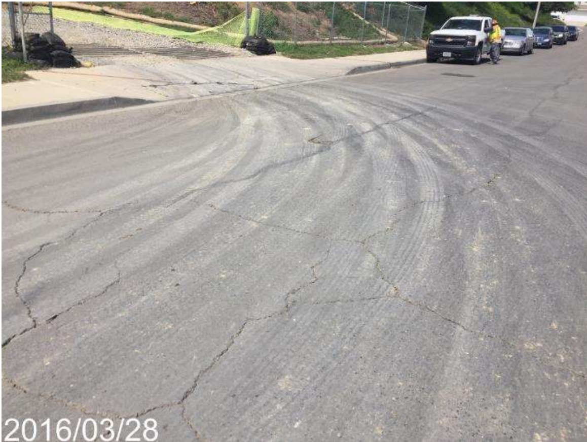
Figure 5: Trackout observed at VC #11, Chino Hills Underground. Photo courtesy of SCE.
